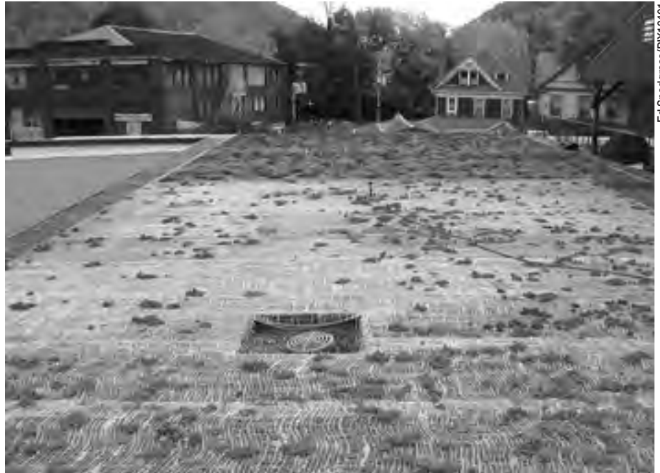
Plants make up a large part of the cost of a green roof. The photo shows establishment using both plant plugs (background) and cuttings (foreground). The plant plugs are forming a dense vegetation cover, whereas the cuttings are developing slowly, leaving most of the soil exposed.
