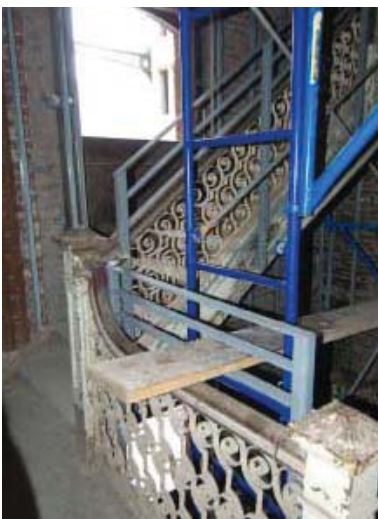
Left: Sample installation of railing modification first proposed did not meet the Secretary's Standards.
