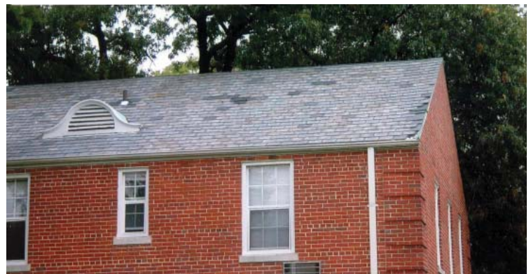
Close up of damaged and previously repaired slate.
