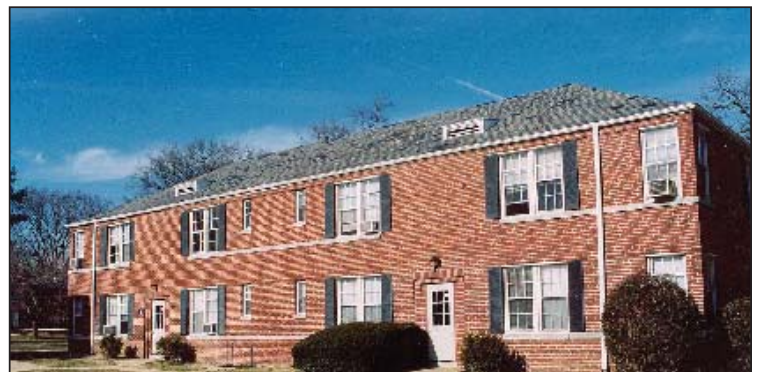
Typical view of Colonial-Revival apartment building in complex before rehabilitation. Note the mottled appearance of original slate due to numerous past repairs.
