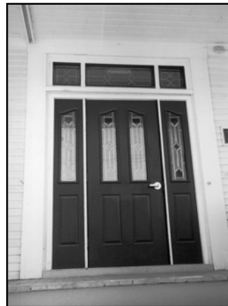
LEFT: Inappropriate replacement entrance.
