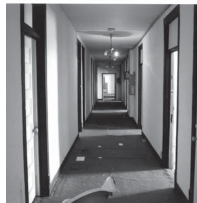
The hotel guest rooms with paneled doors and overhead transoms opened off the double-loaded corridors.
