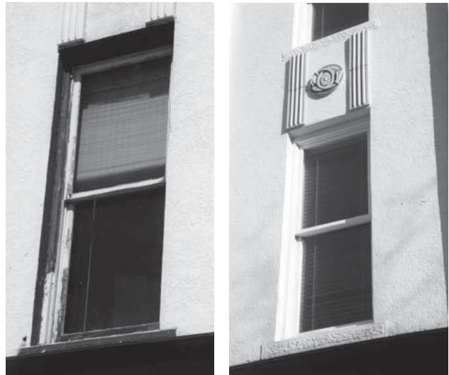
Before/after. Window sash on the street elevations were repaired and retrofitted with a piggyback interior energy panel.
