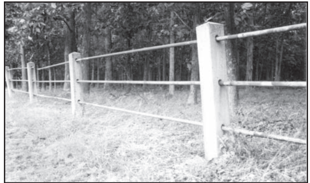
Figure 3.29. Concrete post and iron rail fence on Farm #1 along boundary with Gettysburg NMP, near skeet range, view toward east. (Photo by OCLP, 2002)
