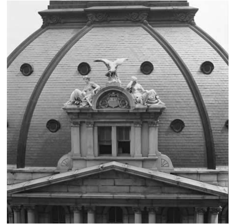
Detail of United States Custom House and Post Office, Saint Louis, Missouri
