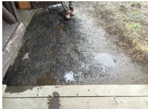
Drainage and access issues at comfort station
