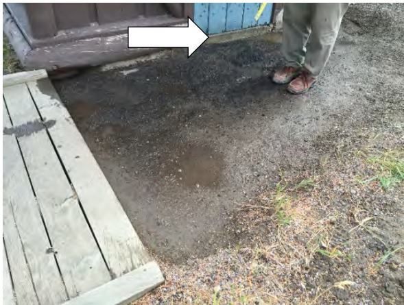
Greater than 1/2" rise at entrance to comfort station
