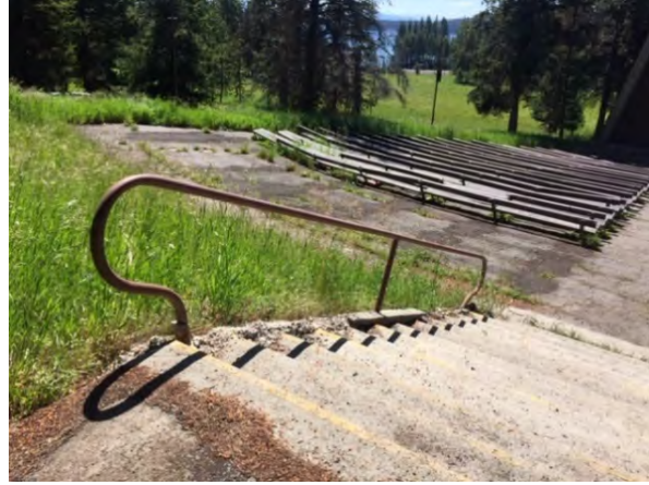
Deteriorated steps and railing to amphitheater seating
