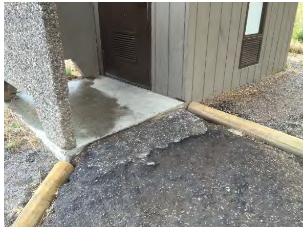
Deteriorated asphalt walkway
