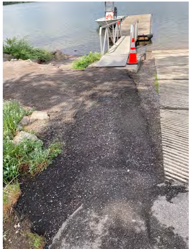
Deteriorated path to gangway
