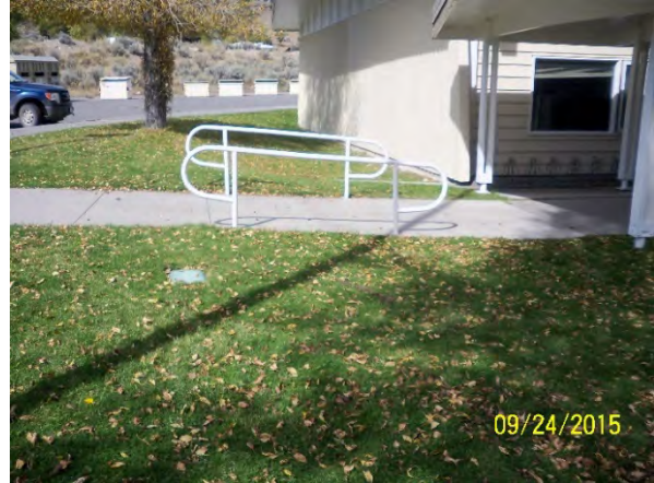
Handrails at entrance to MCC
