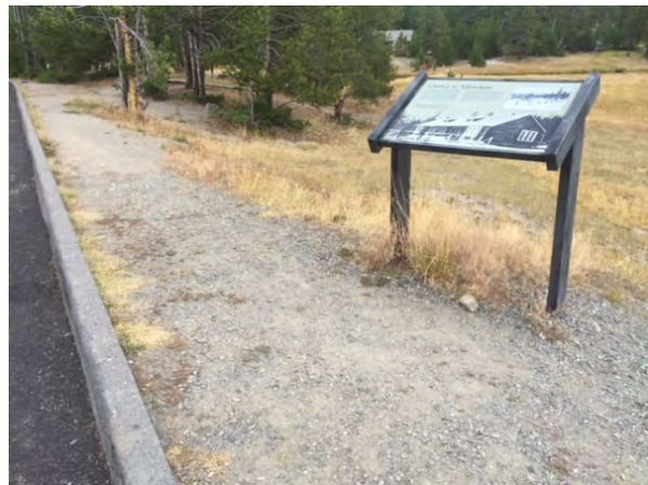
Curb prevents access for users of mobility devices
