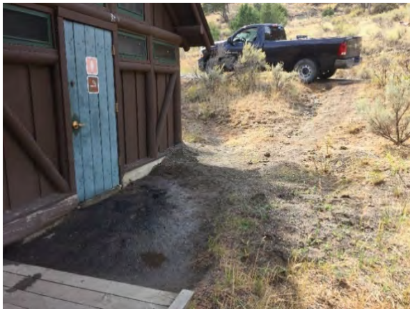
No accessible route to comfort station
