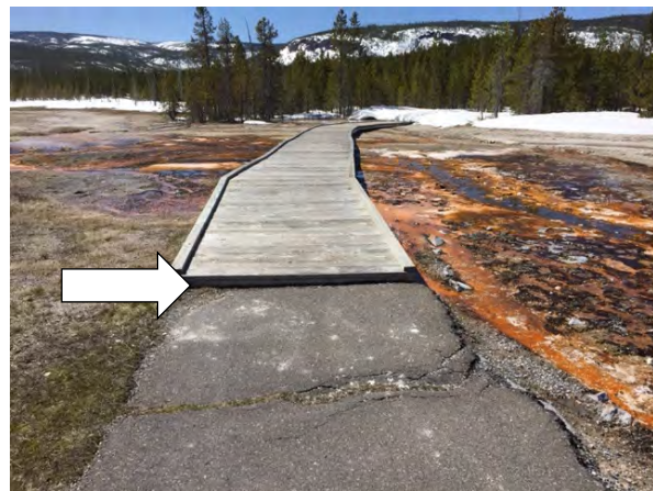
Too much rise between asphalt trail and boardwalk in the Upper Geyser Basin. A large dip and cracked pavement are both safety and accessibility concerns.
