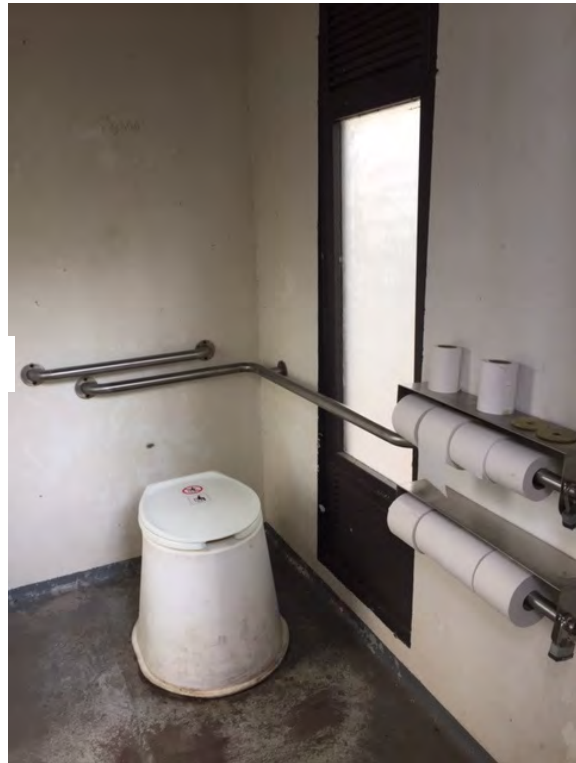
Some grab bars do not meet ABA requirements
