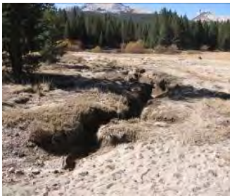
Fig. 1-22. Headcut and downcutting
