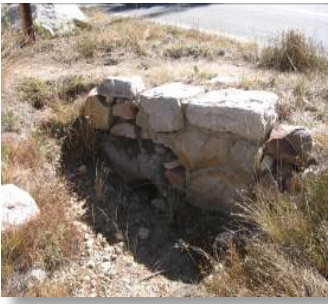
Fig. 1-16. Partially blocked culvert
