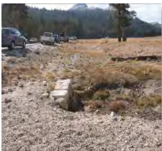
Fig. 1-17. Culvert set too low in meadow
