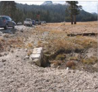
Fig. 1-17. Culvert set too low in meadow
