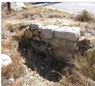
Fig. 1-16. Partially blocked culvert
