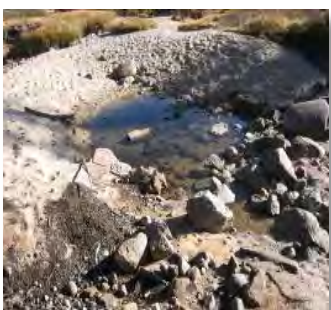
Fig. 1-18. Ponding below culvert at Budd Creek
