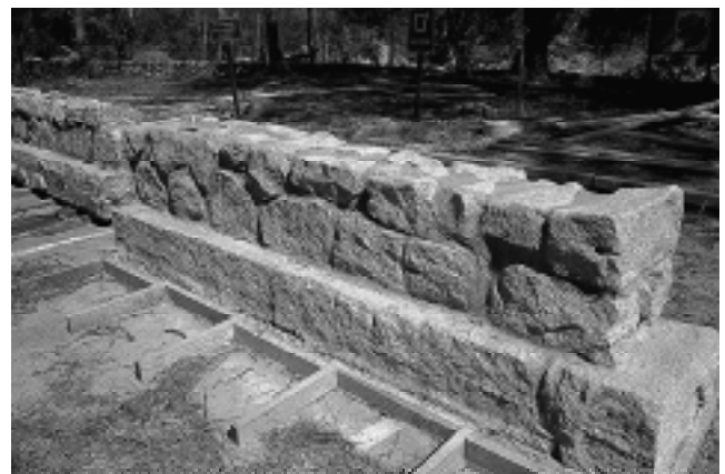
During the proposed reconstruction, the guardwall would be rebuilt. Construction materials still under consideration include molded concrete (formliner, shown here) and a combination of hand-laid granite and formliner.
