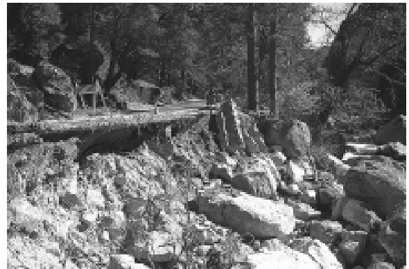
The January flood damaged guardwall, roadbed, and fill slope along the El Portal Road.
