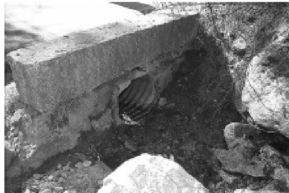
Existing culverts are inadequate in size and number to accommodate flow volume from precipitation.
