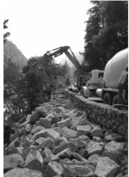
Emergency repair is underway to open the El Portal Road prior to the start of Memorial Day Weekend.
