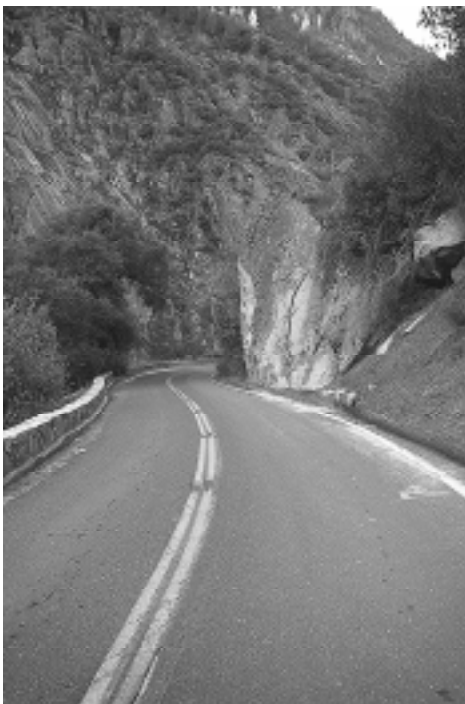
The existing narrow lane width, short line of sight around curves, and close proximity of rock to the pavement make it difficult for drivers to keep vehicles in their lane.
