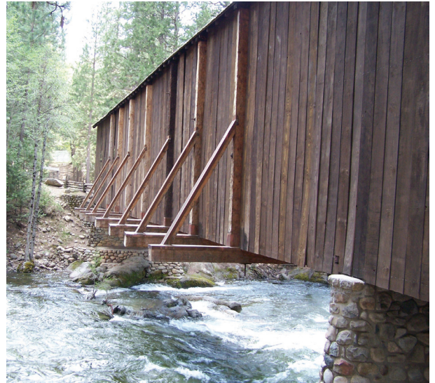
The Wawona Historic Resources ORV, as part of the Merced River Draft Plan, includes one of the few covered bridges in the region.
