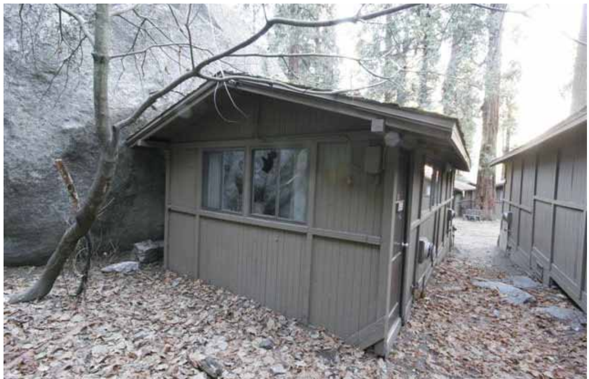
Many of the structures in the realigned rockfall hazard zone were built next to large boulders from previous rockfalls.
