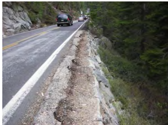
FIGURE 3. FAILURE OF CURB/ROAD SHOULDER
