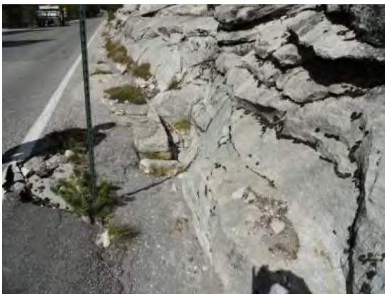
FIGURE 32. EROSION ALONG ROAD SHOULDER
