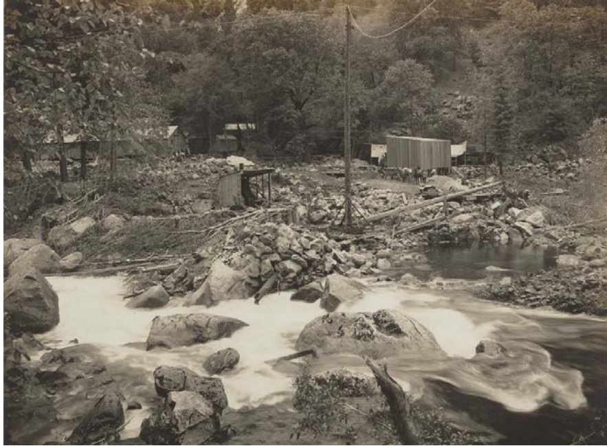
Photo 2.4-13: Before Cascades Diversion Dam Construction (from South Bank)-Undated (taken circa 1916 or 1917, immediately prior to dam construction) (NPS undated)
