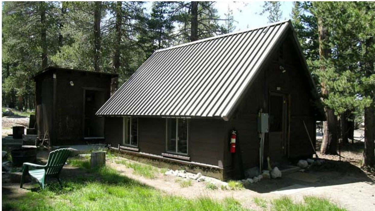
Buildings and Structures #22: View of historic pump house (bldg. #3017), facing northwest. Sump is behind the building. (YOSE, 2006)
