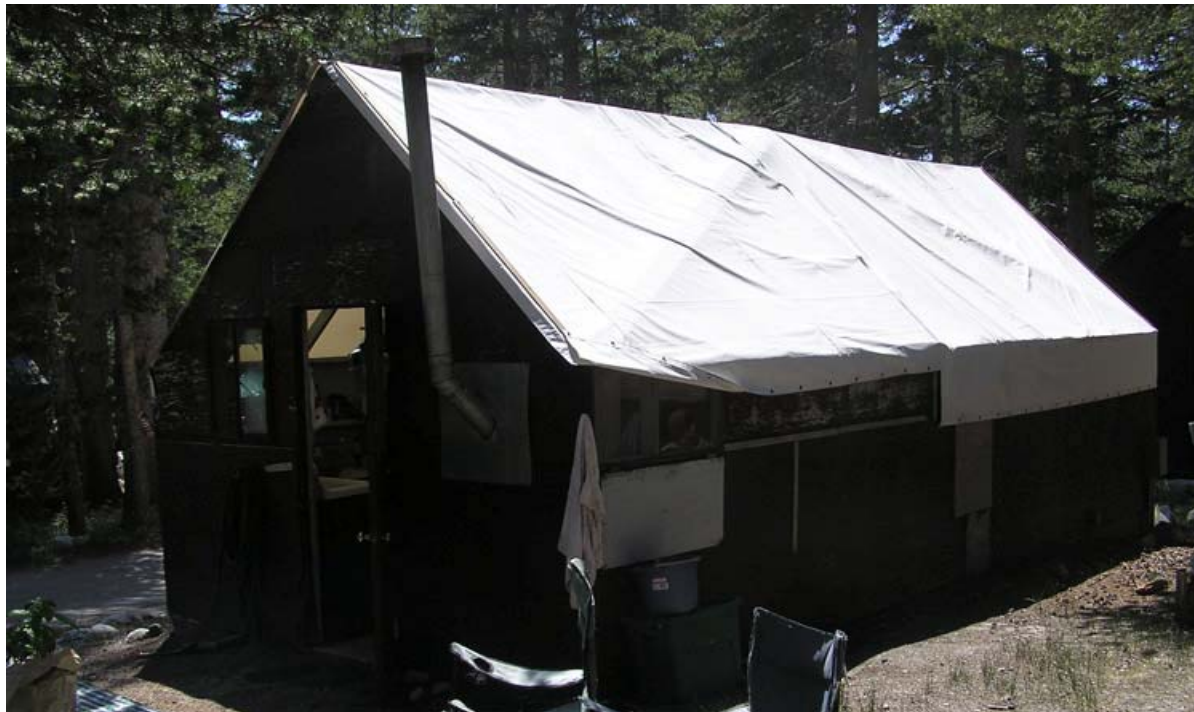
Buildings and Structures #8: View of one of the 5 original tent cabins (bldg. #3032), facing southwest, in the Administrative Area. (YOSE, 2006)
