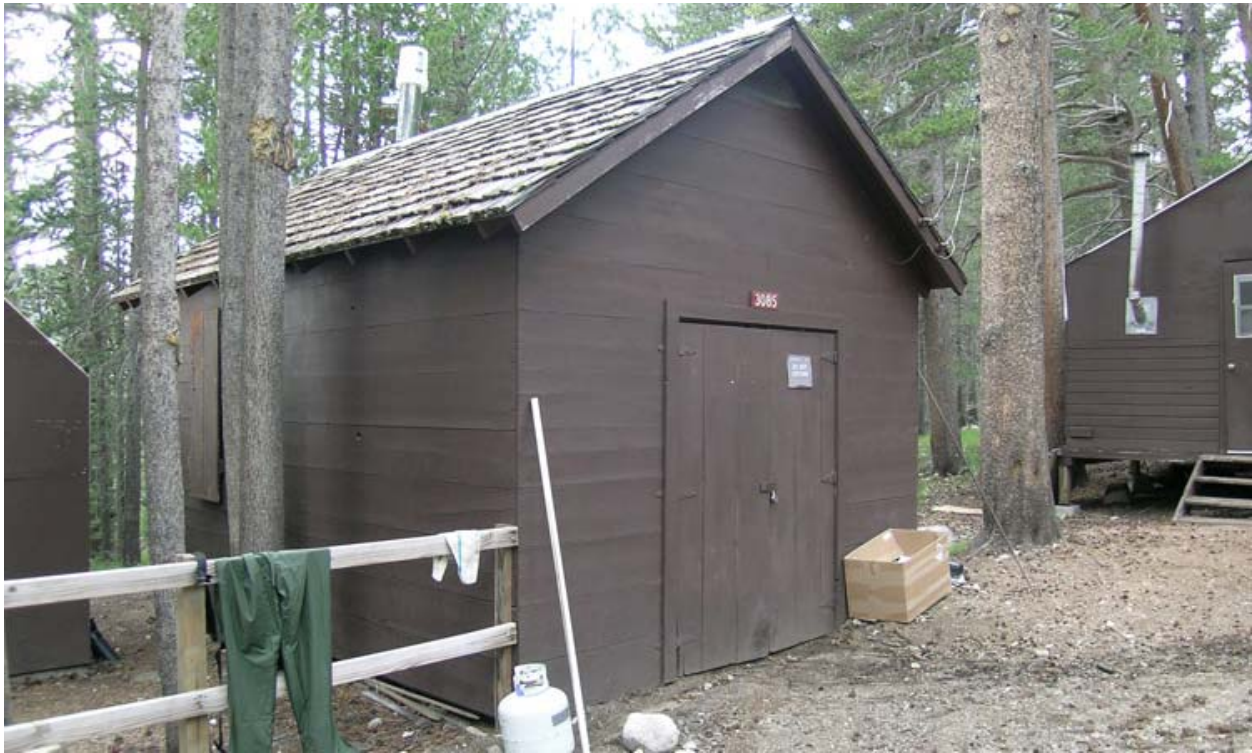
Buildings and Structures #11: View of the storage shed/office (bldg. #3085), facing south, located at the Insect Research Station. (YOSE, 2006)
