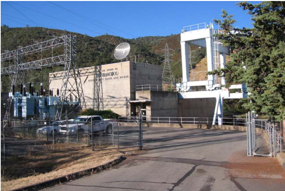
Southeast-facing view of Moccasin Powerhouse Figure 3.10.2-2
