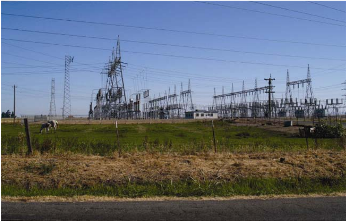
North-facing view of Warnerville Switchyard from Warnerville Road Figure 3.10.2-1
