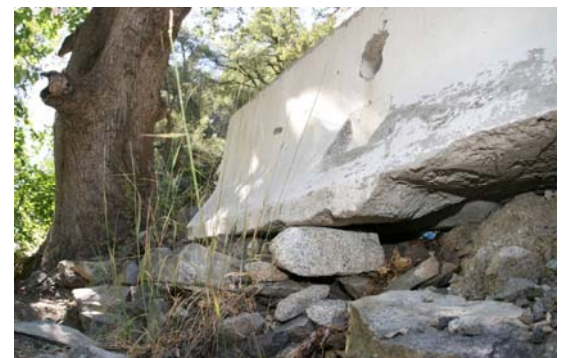
A portion of the undercut roadway bank.
