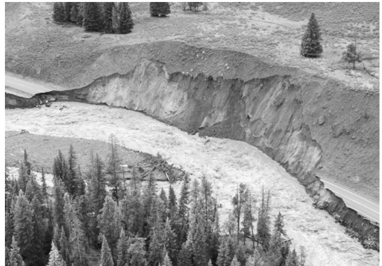
One of many washouts on the Northeast Entrance Road from Tower-Roosevelt to Cooke City, MT.
