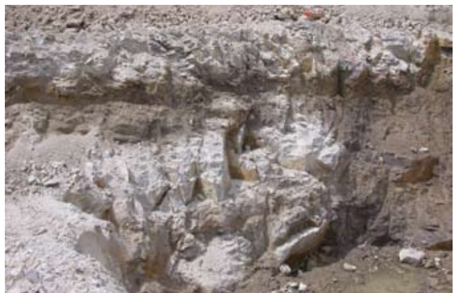
Figure 9. Natural fractures exposed in an excavation for the Norris wastewater treatment plant, June 2004. Notice the near-vertical natural fractures, the spacing of fractures, and the hydrothermally altered fracture surfaces of the Lava Creek B tuff. Dark colors show moist zones within the outcrop.
