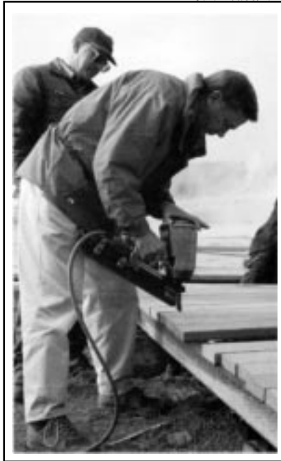
Above: Secretary of Interior Bruce Babbitt trying out the fastening system on the recycled boardwalk.
