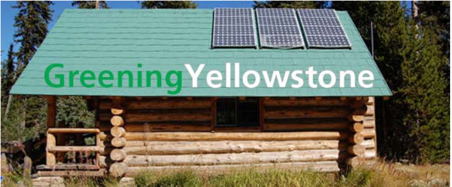
Solar panels provide power at the Lewis Lake Contact Station.
