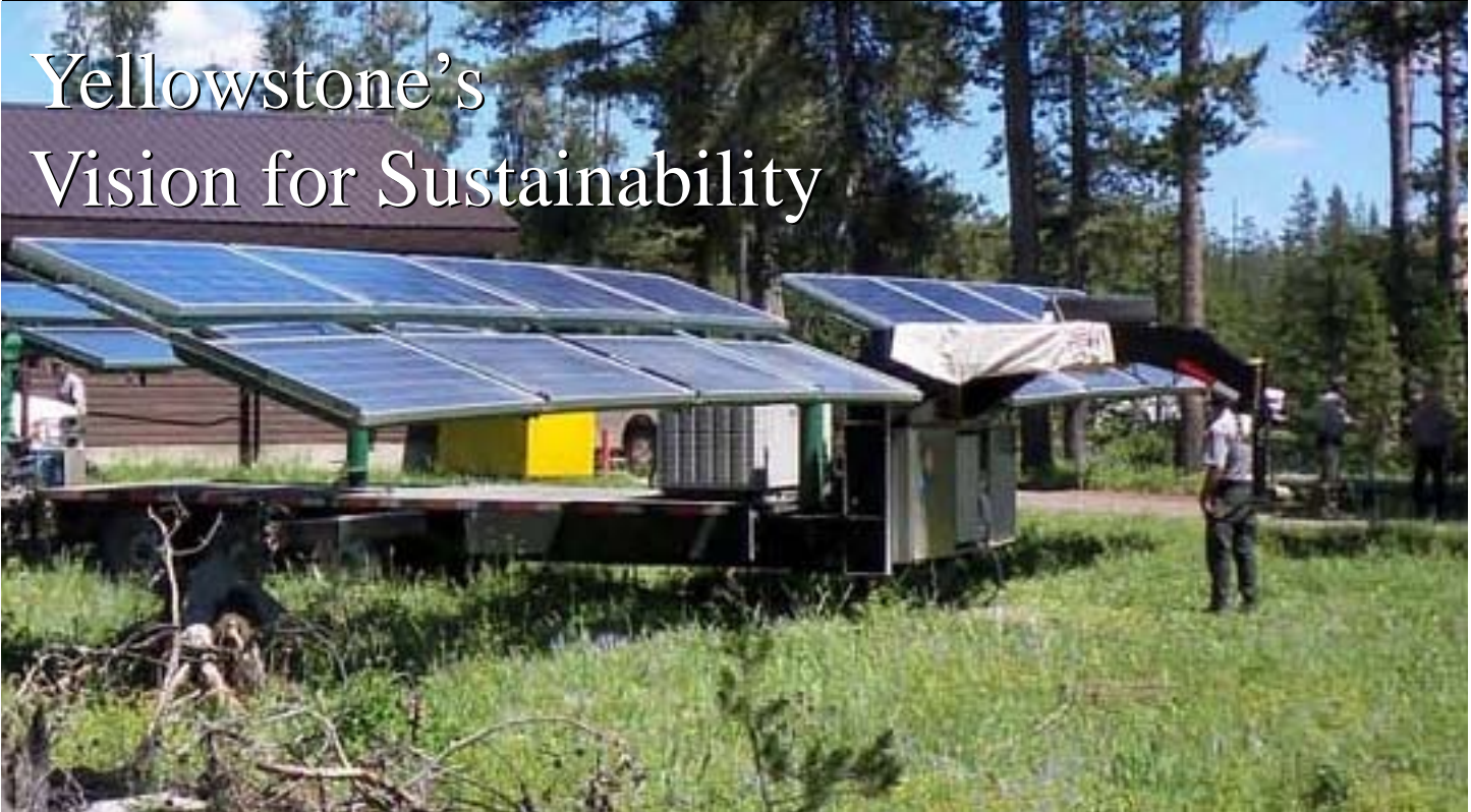
A portable solar array provides power at the Bechler Ranger Station in the summer season.
