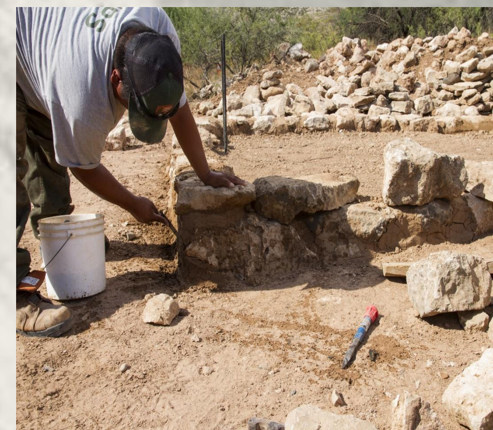
Using a tuck pointer to push in the mortar. During the construction of the Replica pueblo.
