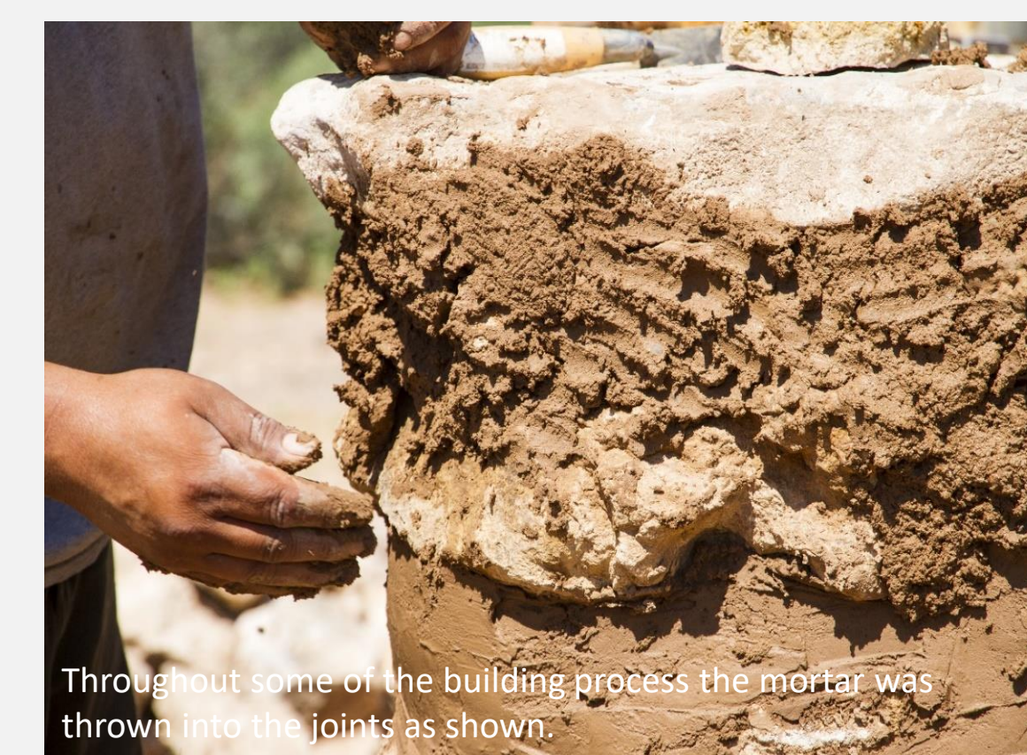
Throughout some of the building process the mortar was thrown into the joints as shown.
