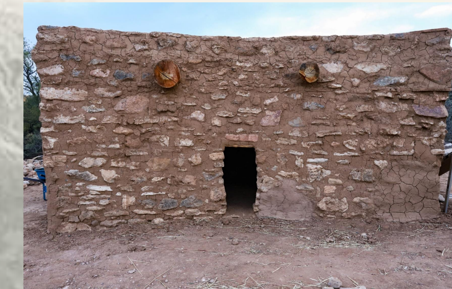
Prior to any plastering, many tests were conducted. Notice the two test patches at the east side of the entrance and at the corner.
