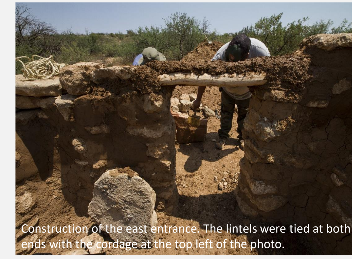
Construction of the east entrance. The lintels were tied at both ends with the cordage at the top left of the photo.
