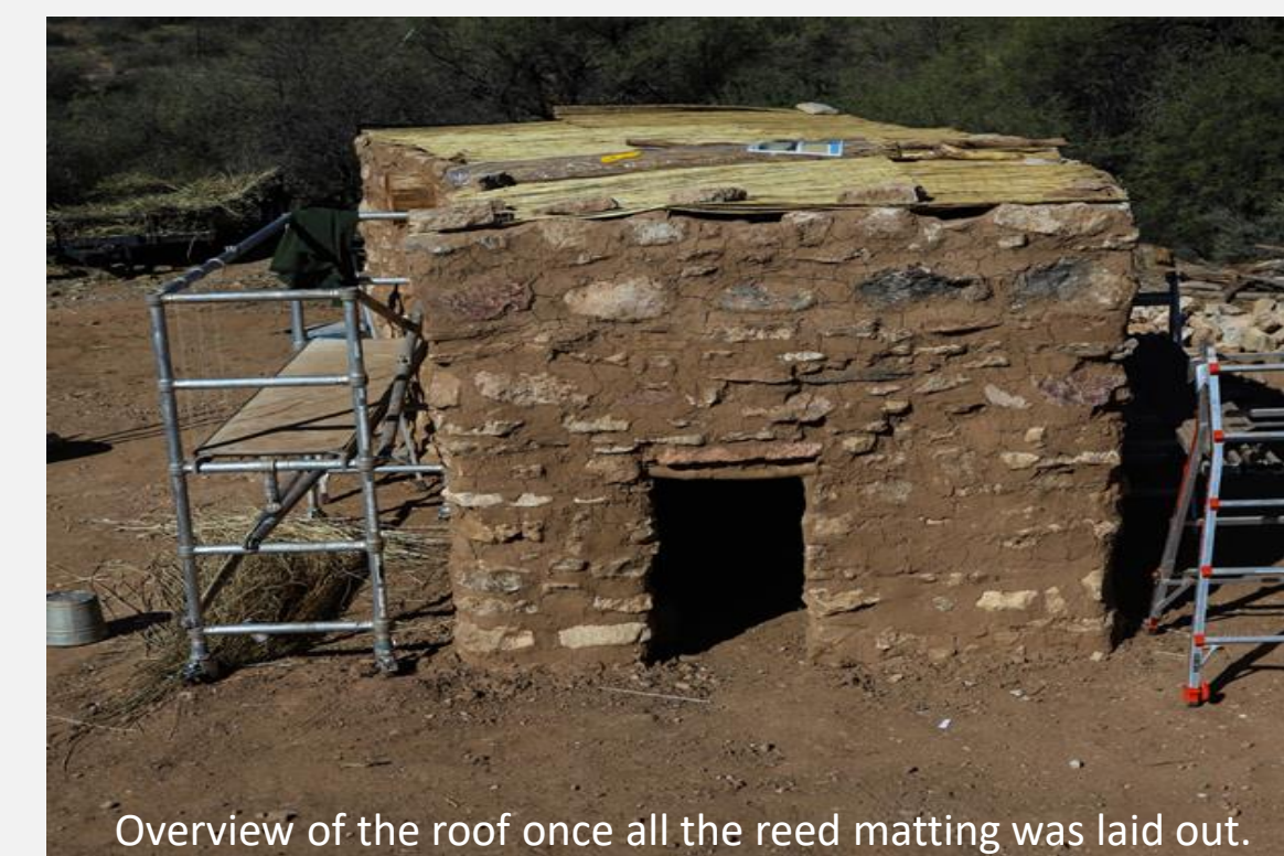
Overview of the roof once all the reed matting was laid out.
