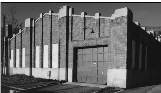
Just prior to rehab, the existing garage door was a single wood roll-up style, divided into thirty segmented solid panels by intersecting stiles and rails.
