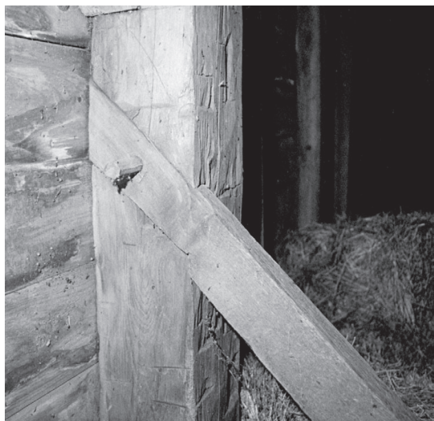
Through-lapped half-dovetails are common. The through housing removes more wood from the post than a stopped housing, but it can be sawn to full depth, saving considerable chiseling work. The dovetail slope typically is cut on the inward-facing edge of the brace. This brace runs from a post down to a tie beam in a scribe rule German barn dismantled in Alcove, New York, and moved to Long Island.
