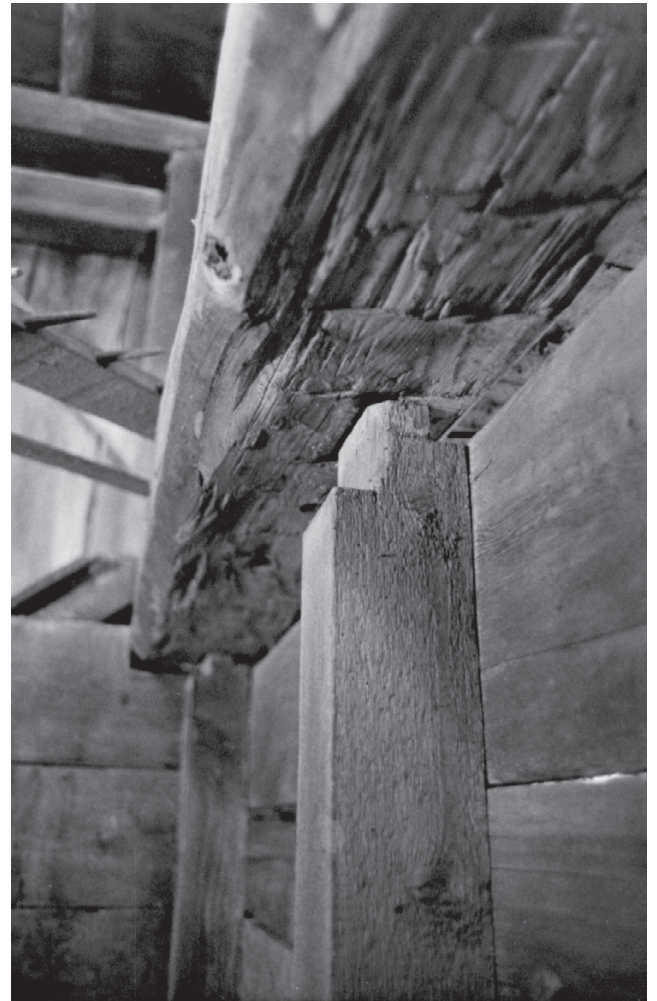
This partially withdrawn stud in a barn in Shaftsbury, Vermont, was relieved at its end to make its tenon barefaced. Uncommonly, the relief cut was not angled, and gives the appearance of a second cheek and shoulder.
