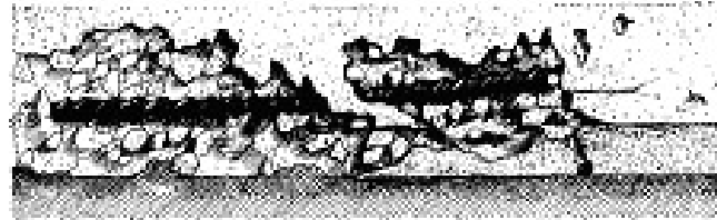
Battery Marcus Miller: Detail view of spalling concrete. Spalling can be caused by expansive corrosion acting on reinforcing steel
