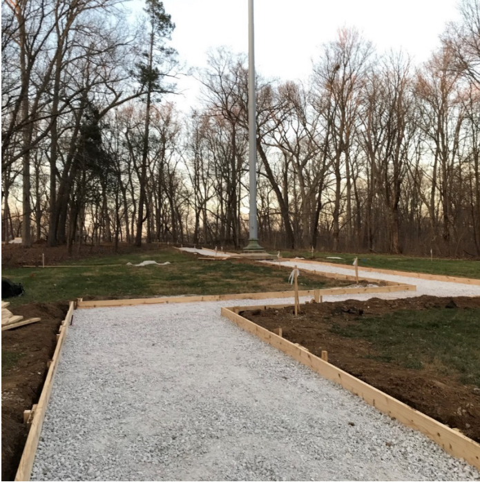
Figure 14. Trail to the flagpole terrace and cemetery are framed in wood forms and ready for the concrete pour. (NPS/Rhonda Schier)
