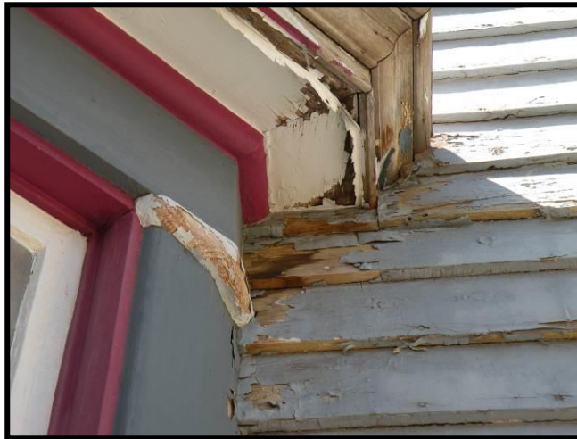
Figure 4.11. Coating failure near the end grain in an area where water flowed down the face of the exterior cladding, as evidenced by the moisture stains on the exposed wood.
