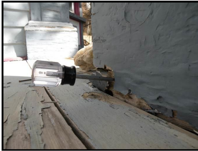
Figure 4.18. Probing at the base of a porch column with an awl reveals some deterioration.
