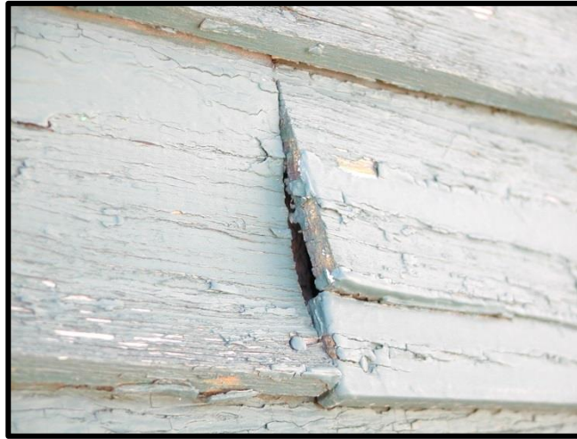
Figure 5.3. Cupping and splitting of boards on a historic theater building.
