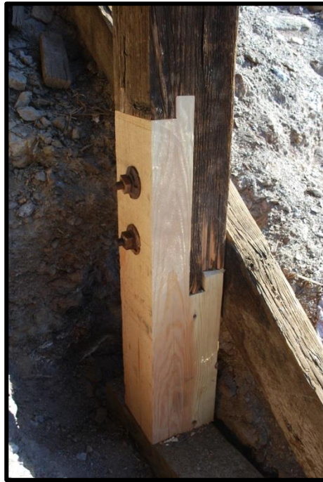
Figure 5.6. A Dutchman repair on an exterior column that had deteriorated in ground contact (courtesy of Douglas Porter, Conservation Associates).
