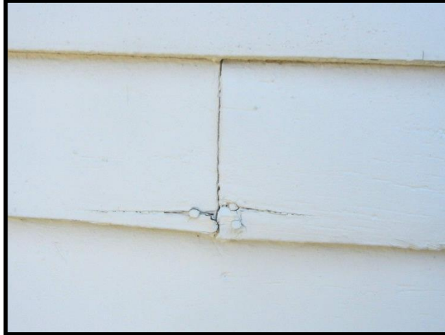
Figure 5.4. Horizontal siding with a butt joint. Note the siding has also been face-nailed in an attempt to prevent or minimize cupping. Face nailing tends to lead to board failure, as the wood is forced to move differentially, leading to splits, as shown here.
