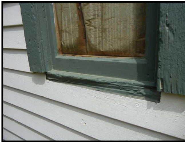
Figure 4.17. Missing window sill.
