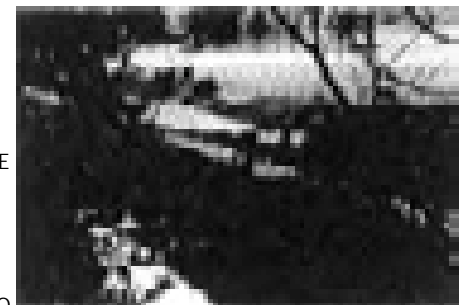
ARREST EROSION. THE USE OF NATIVE STONE ASSISTS IN MAKING GABLONS A VISUAL COMPLEMENT TO THE NATURAL ENVIRONMENT.
