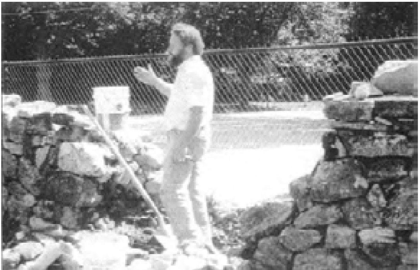
A section of a historic wall at Stan Hywet Hall in Akron, Ohio, was in need of restoration. Here, the limited replacement of a section of the wall was undertaken utilizing surviving stone and stones that matched the old in form, size, and color. Compatible substitute material could also have been used. (author, 1993)
