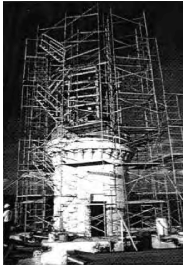
Restoration of the lighthouse tower at Las Cabezas de San Juan in Faiardo, PR (1990)
