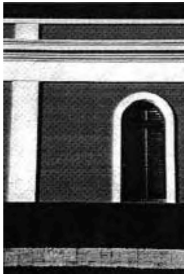
Detail of side facade showing final result of compatible finishes for plasters and lime washes. Lighthouse at Las Cabezas de San Juan in Fajardo, PR (1991).
