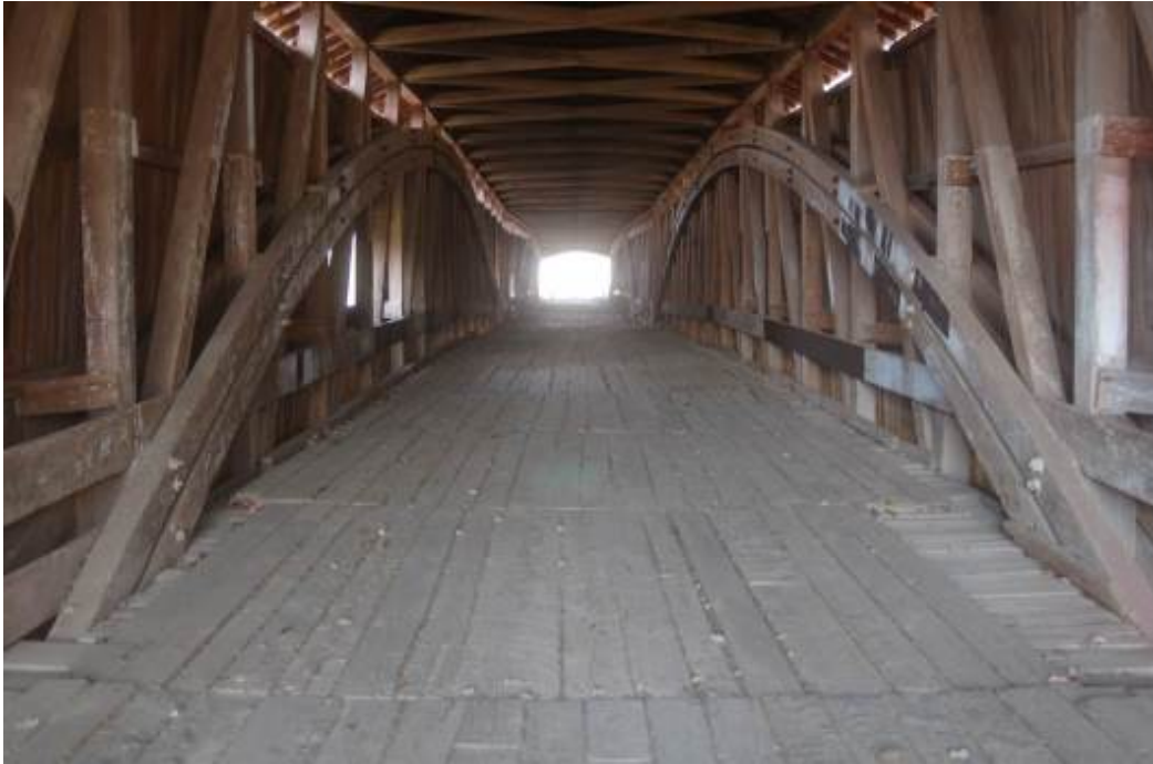
WEST UNION BRIDGE. Interior view looking toward south portal. Photograph by Lola Bennett, 2015.
