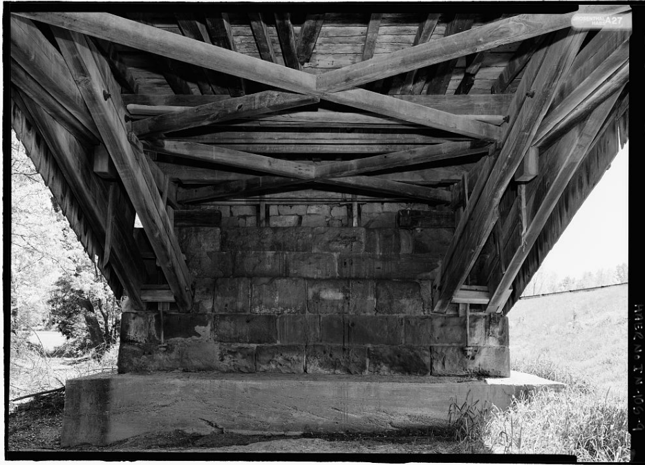
WEST UNION BRIDGE. Elevation of south abutment. Photograph by James Rosenthal, 2004 [HAER No. IN-105-9].
