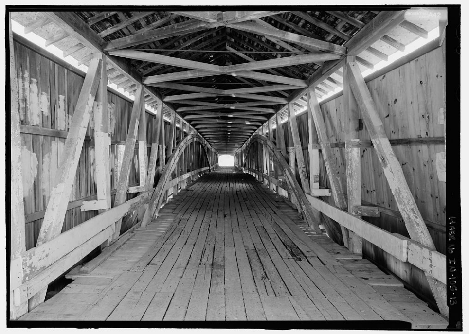
WEST UNION BRIDGE. General view of interior from north. Photograph by James Rosenthal, 2004 [HAER No. IN-105-13].
