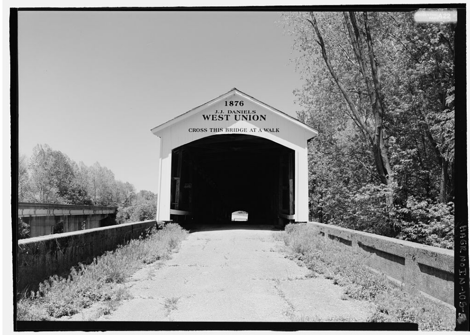
WEST UNION BRIDGE. South portal elevation. Photograph by James Rosenthal, 2004 [HAER No. IN-105-4].
