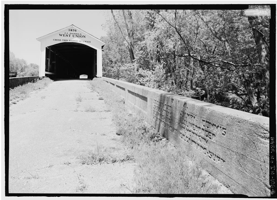
WEST UNION BRIDGE. View of 1914 concrete approach. Photograph by James Rosenthal, 2004 [HAER No. IN-105-6].
