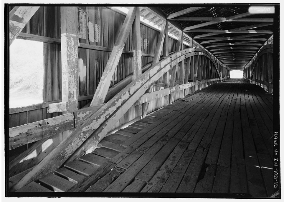
WEST UNION BRIDGE. Oblique view of arch from north. Photograph by James Rosenthal, 2004 [HAER No. IN-105-15].
