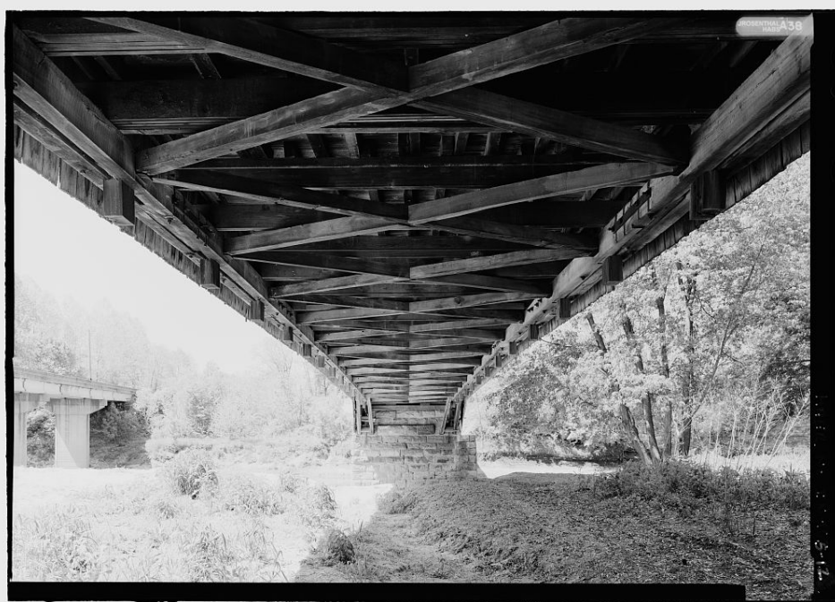
WEST UNION BRIDGE. View of floor system from south. Photograph by James Rosenthal, 2004 [HAER No. IN-105-12].
