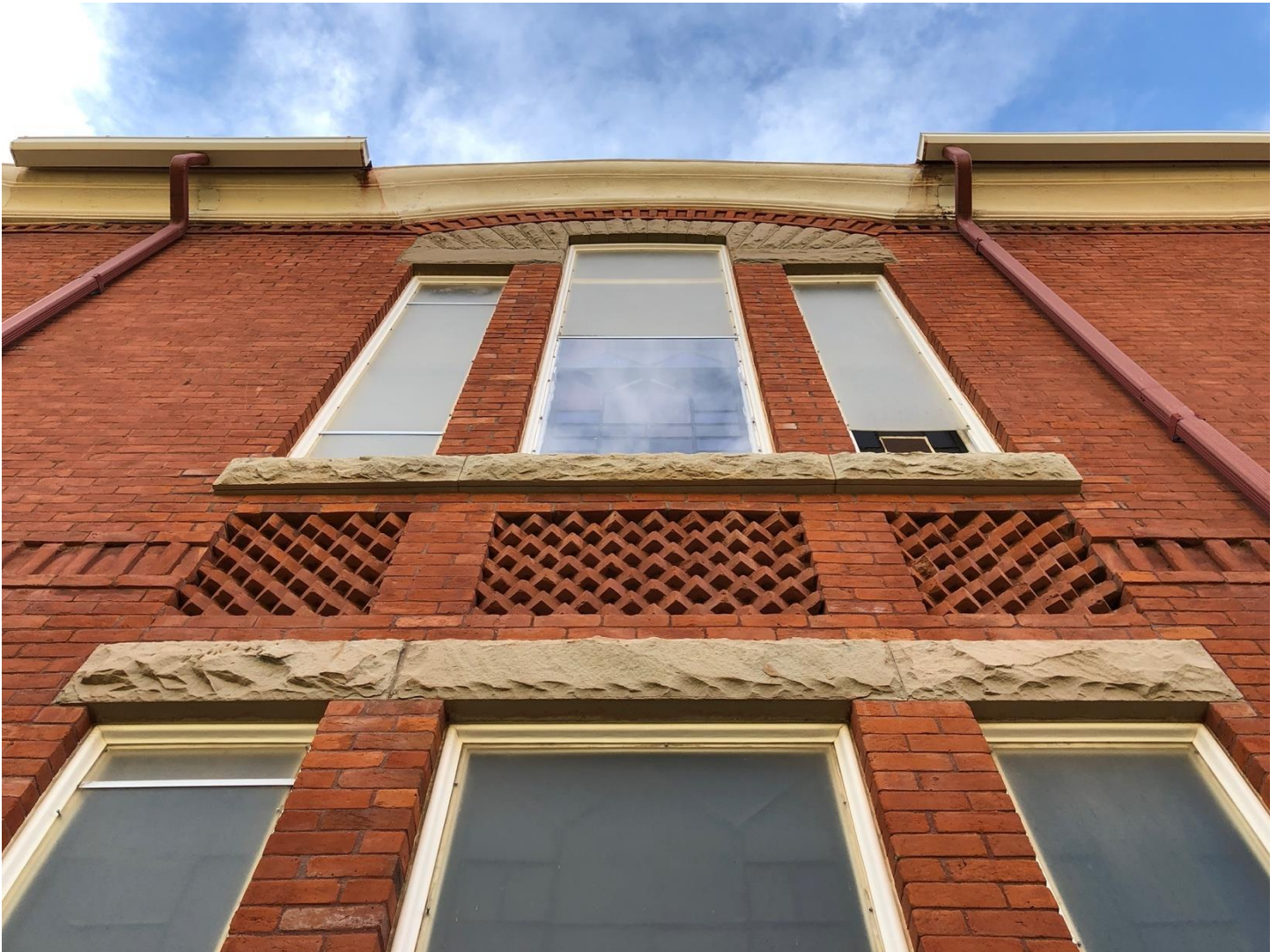
Photo 4 of 39. Temple Aaron, south side, detail of tripartite window arrangements, stone lintels and sills, decorative brick panels, and dentilated brick, view west-northwest.
