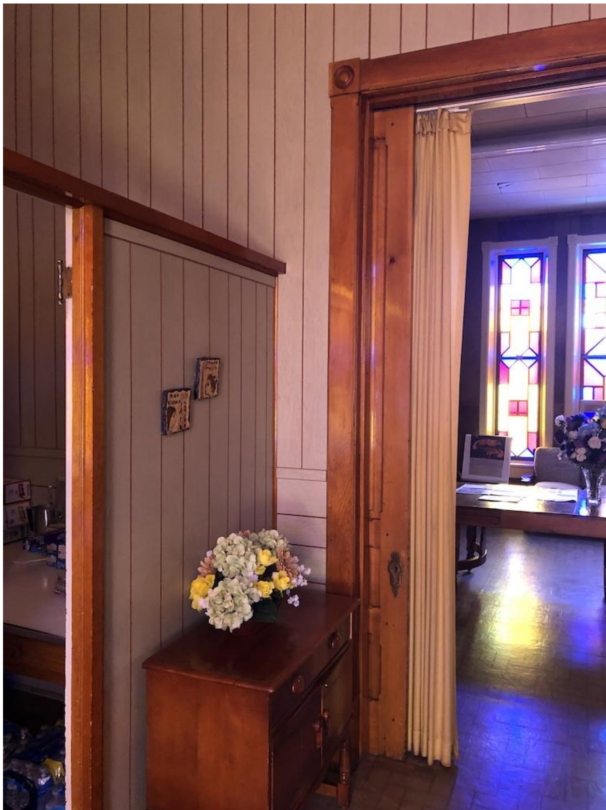
Photo 19 of 39. Temple Aaron, view of paneled kitchen partition wall and pocket door opening into north classroom.
