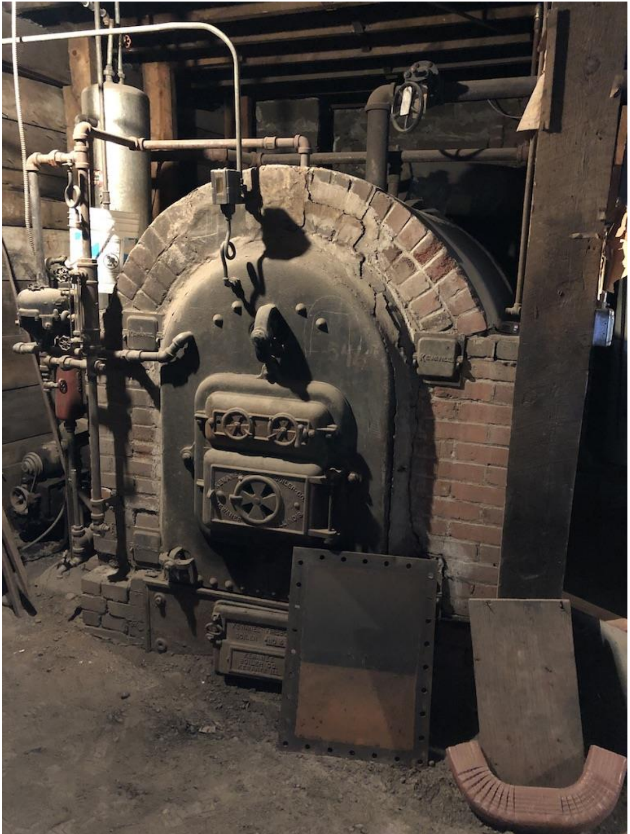
Photo 34 of 39. Temple Aaron, basement, original boiler manufactured by the Kewanee Boiler Company in Kewanee, Illinois.
