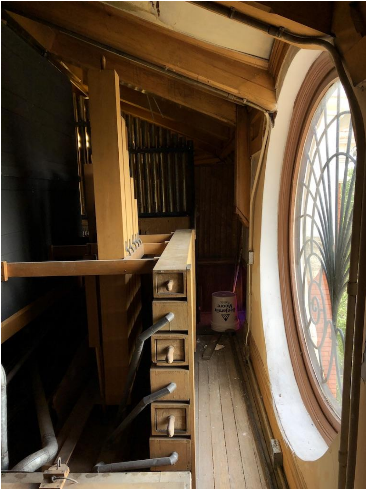
Photo 32 of 39. Temple Aaron, rear of organ in front of the central circular window with decorative iron grille.
