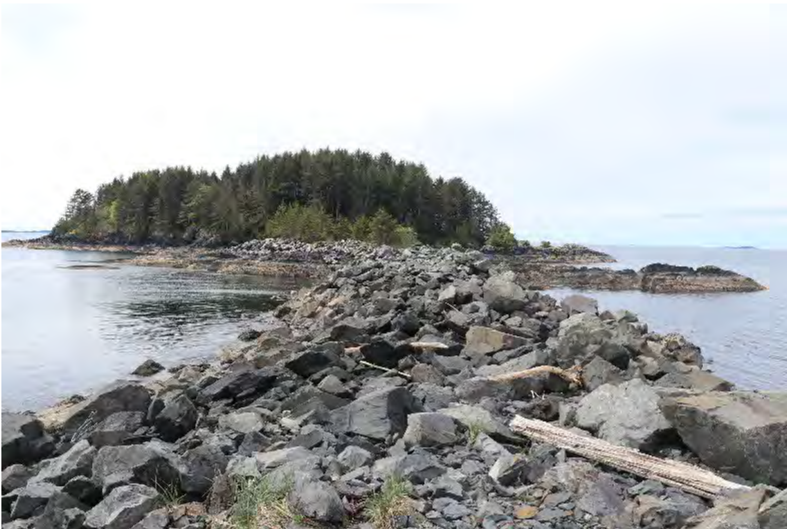
Photo 22 of 43. Causeway between Makhnati Island and Mogilnoi Island, view is southwest from Mogilnoi, May 2022. Note bare armor rock with no gravel on top.
