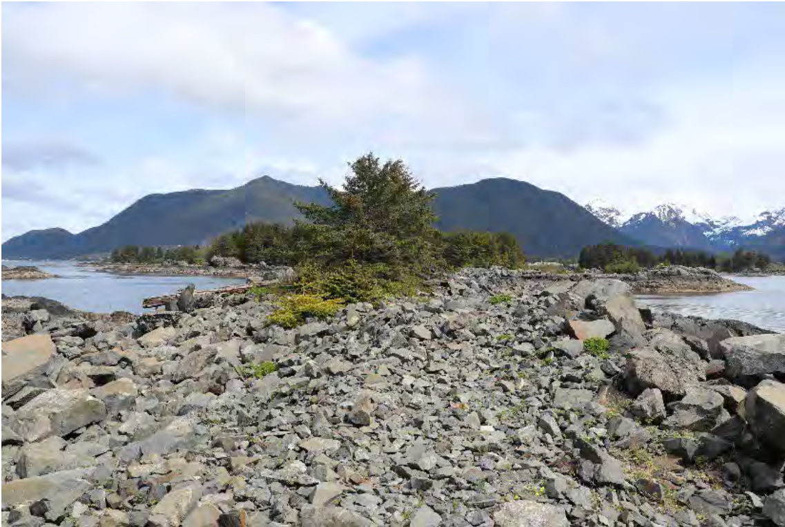
Photo 21 of 43. Causeway between Makhnati Island and Mogilnoi Island, view is northeast from Makhnati, May 2022. Note bare armor rock with no gravel on top.
