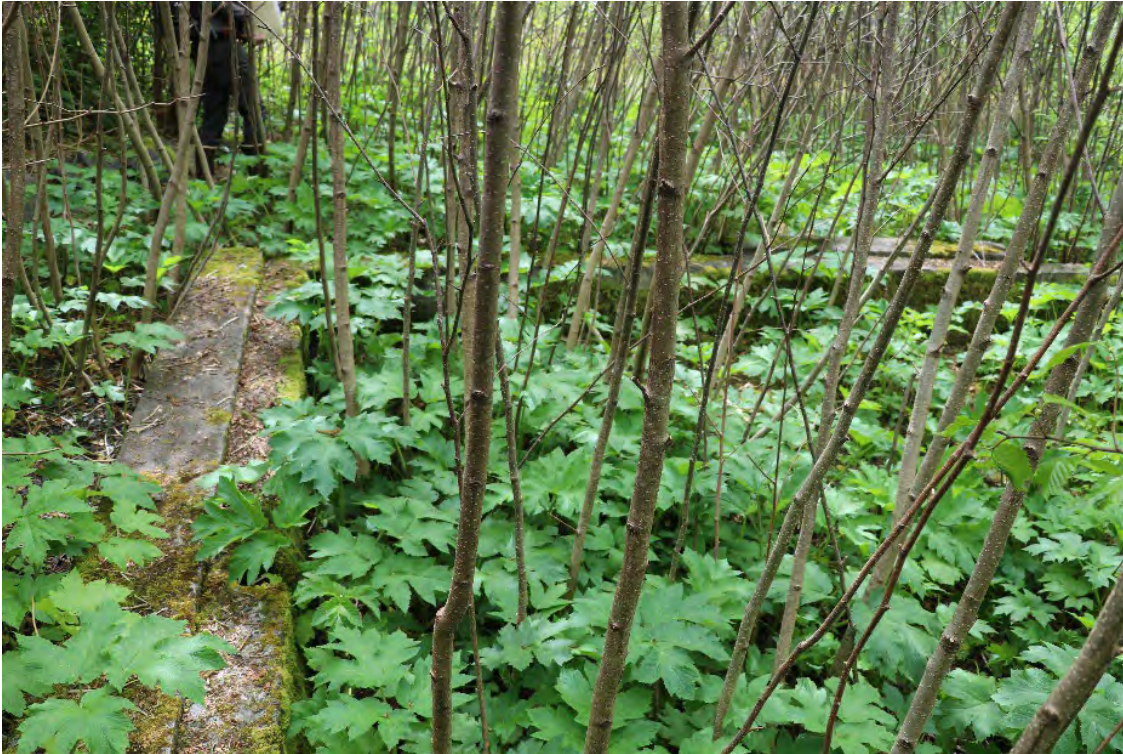
Photo 32 of 43. Foundation just south of entrance to the Gold Island Bunker (possibly to the former fuse house), view is south, May 2022.
