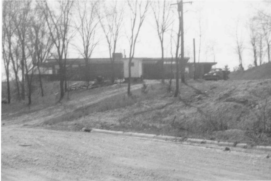
Fig. 1 Samara under construction, 1955. View from Woodland Avenue. Courtesy the John E. Christian Family Memorial Trust.
