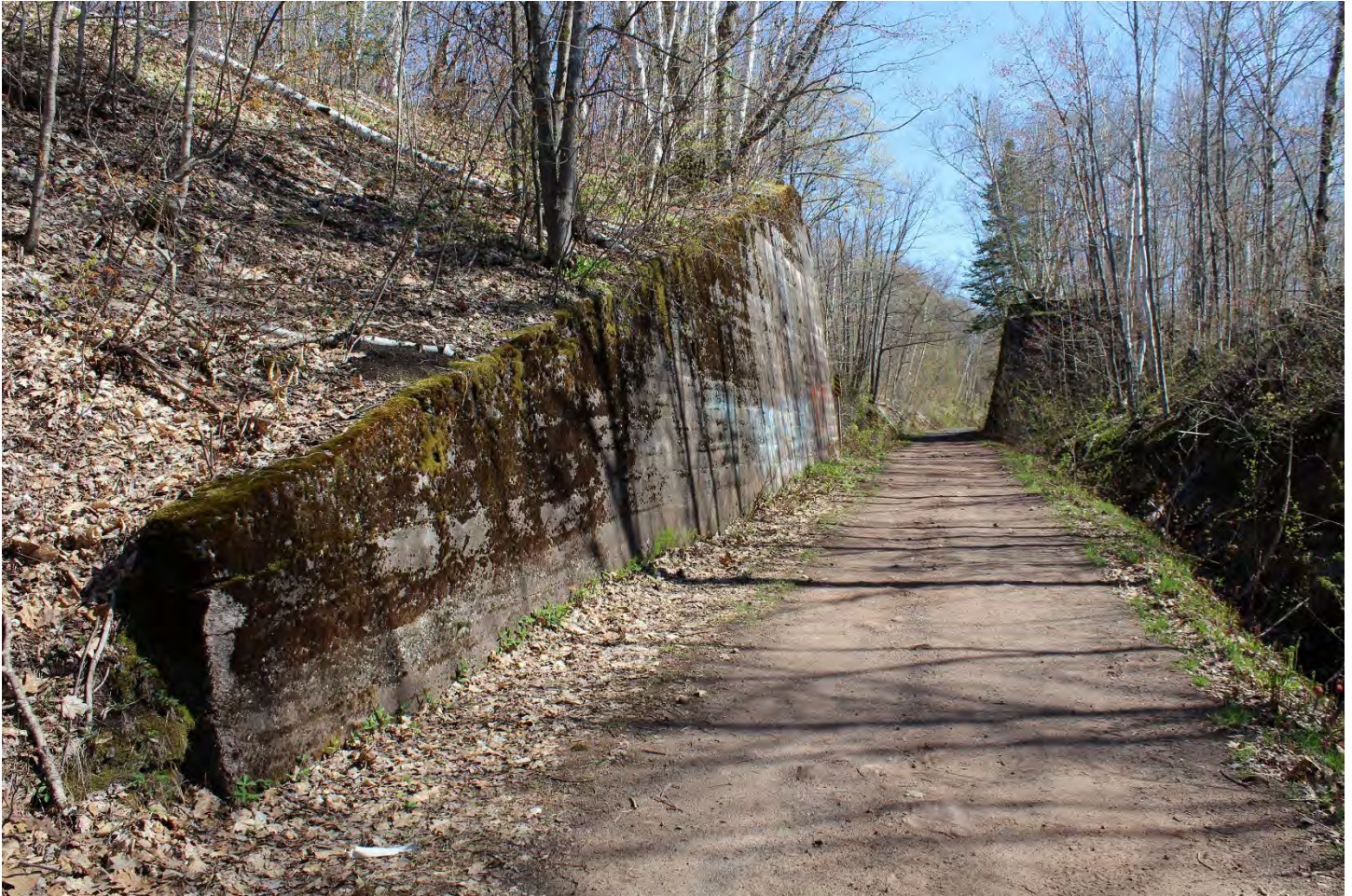
Quincy and Torch Lake Railroad Corridor, Landscape Character Area 6. Detail of retaining walls along the corridor.
