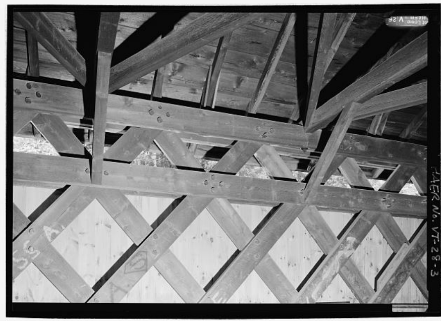
BROWN BRIDGE. Connections, upper chord, north truss. Photograph by Jet Lowe, 2004 [HAER VT-28-3]
