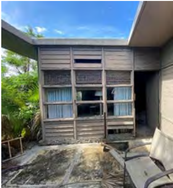
Figure 7 - Return Wall in Poor Condition
