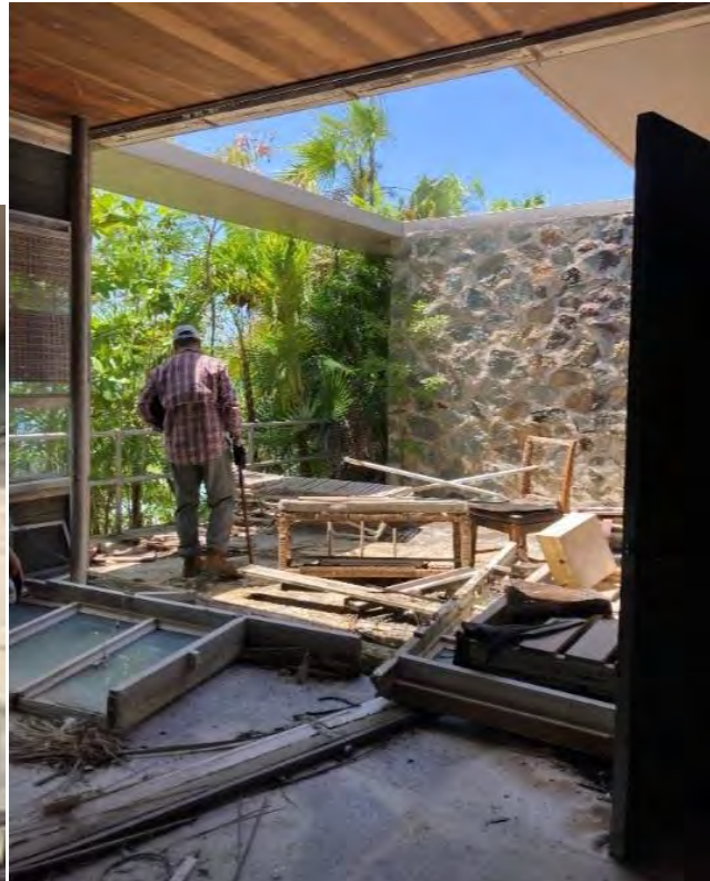
Figure 8 – Failed Return Wall
