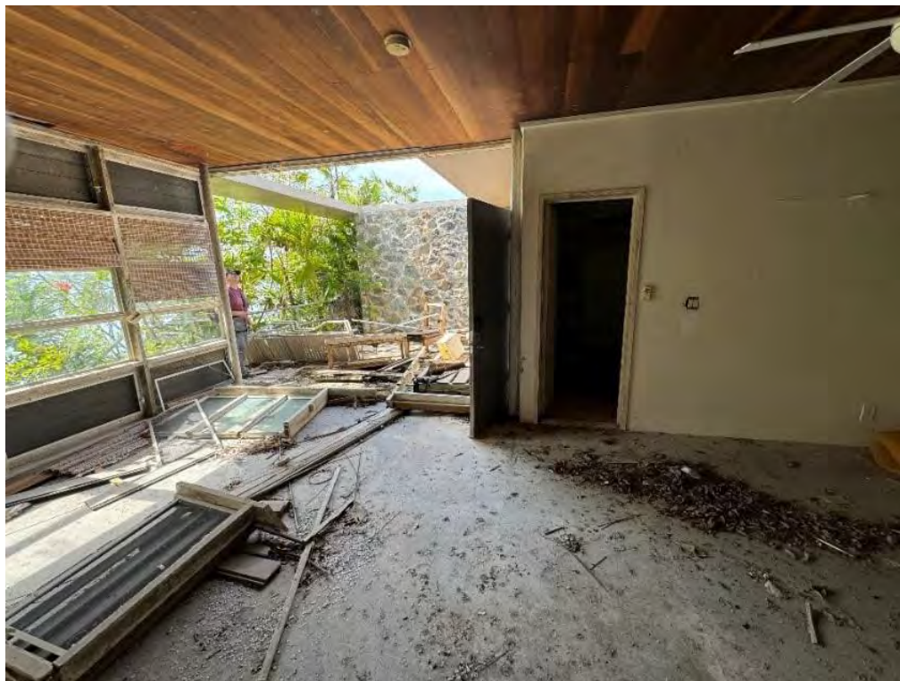
Figure 2 - Failed Return Wall
