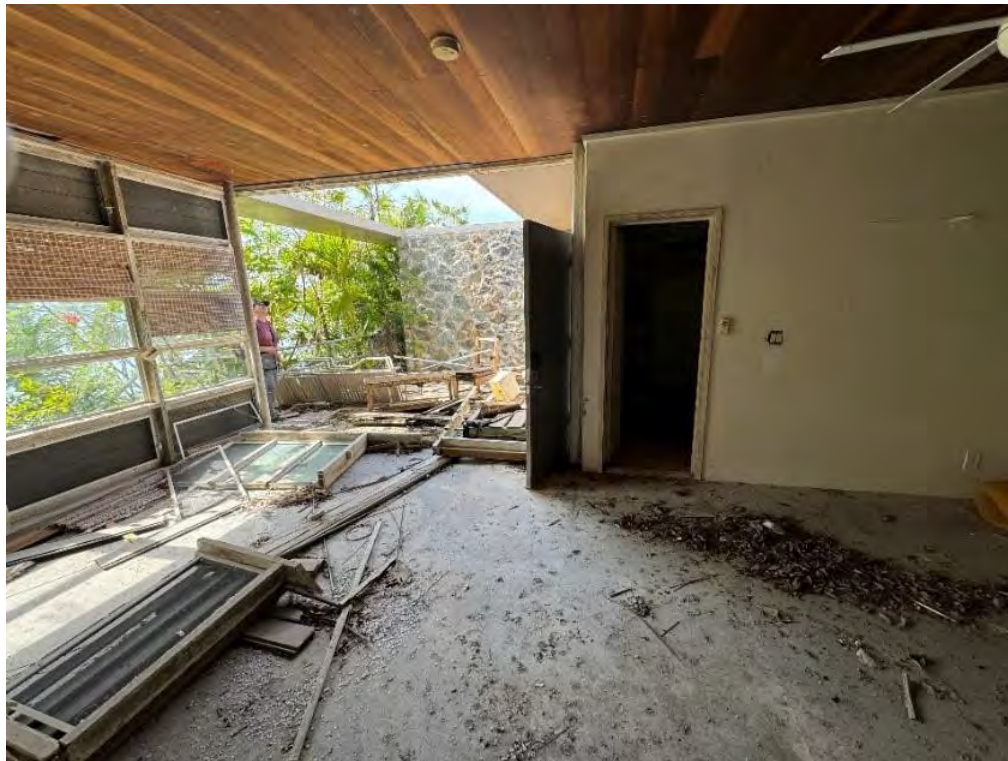
Figure 2 - Failed Return Wall
