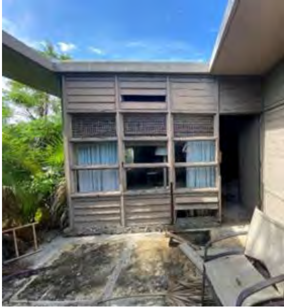
Figure 7 - Return Wall in Poor Condition
