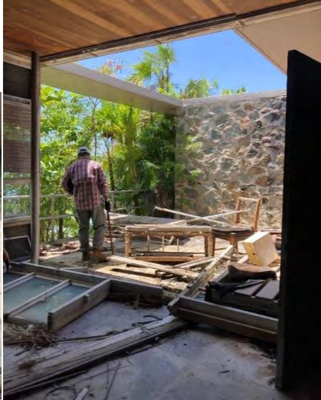
Figure 8 - Failed Return Wall
