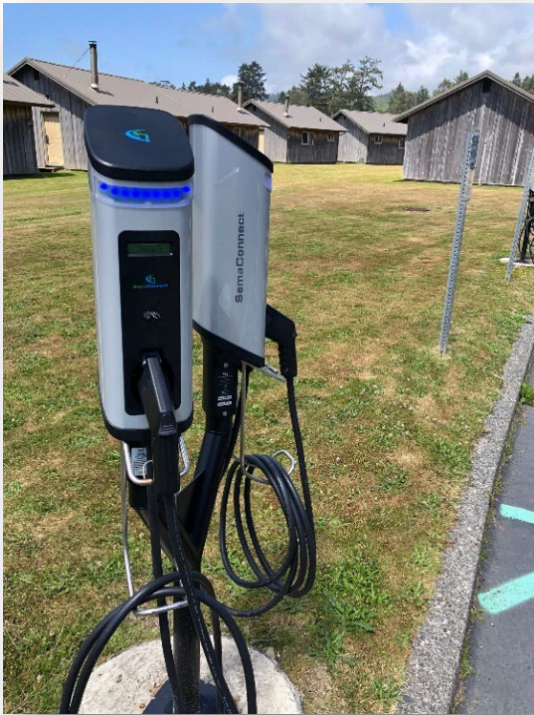
EV Charging Station, National Park Service
