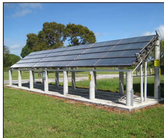
Solar arrays provide hot water at Flamingo campgrounds. NPS Photo
