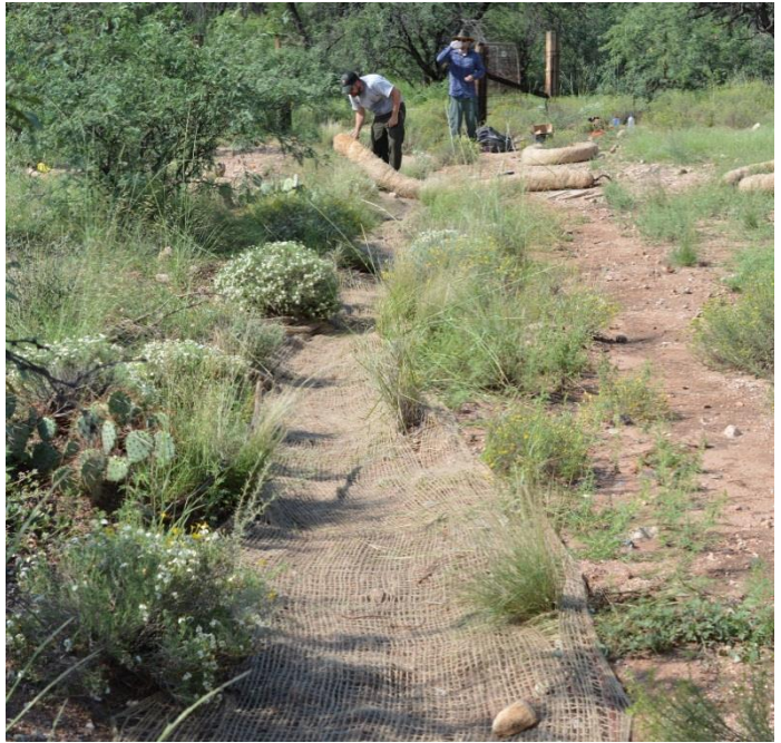
Figure 4. Jute matting (foreground) has just been placed over the erosion channel. Cultural resource staff is preparing to install excelsior waddles (background).
