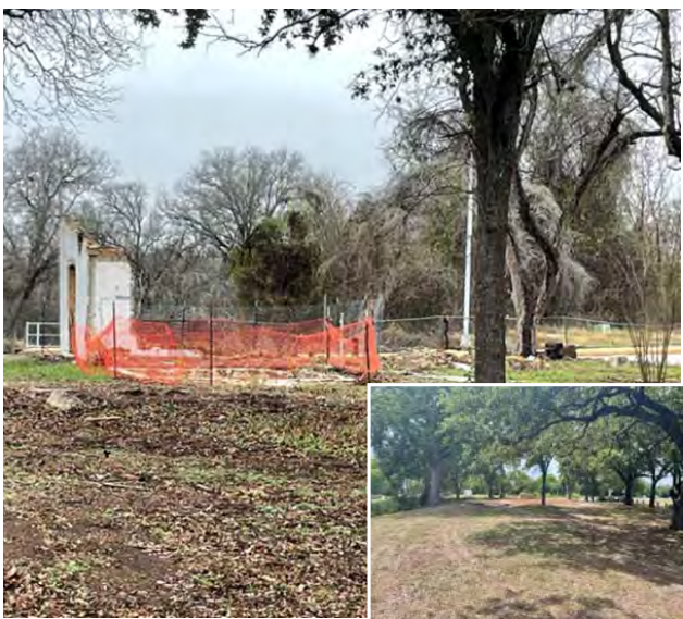
Before and after demolition and cleanup of the Sisson House by Mission San Juan.
