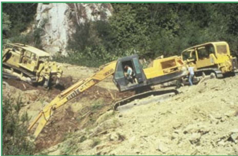
Geologists and heavy equipment operators work together as a team to ensure that they leave a naturally functioning ecosystem after road removal.
