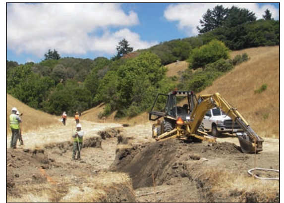
To stem the infusion of sediment and pollutants into the watershed, crews repaired and filled in the Truttman Ranch Headcut.
