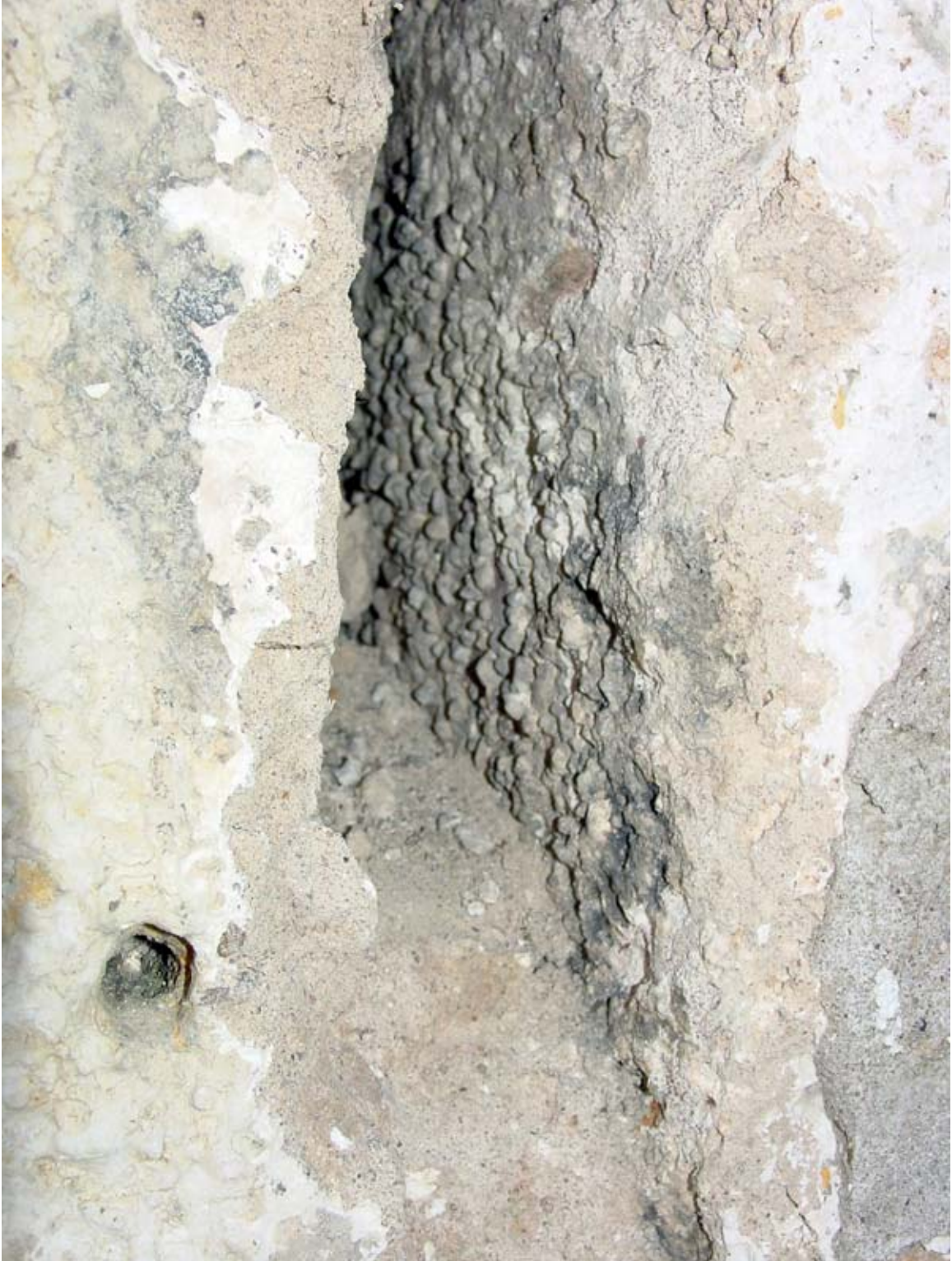
Photo NEd - Detail view of seam at north elevation between main block (right) and east addition (left), looking south. Note textured surface of stucco and that stucco wraps around east side of the main block. View represents the general location of Material Sample 26.
