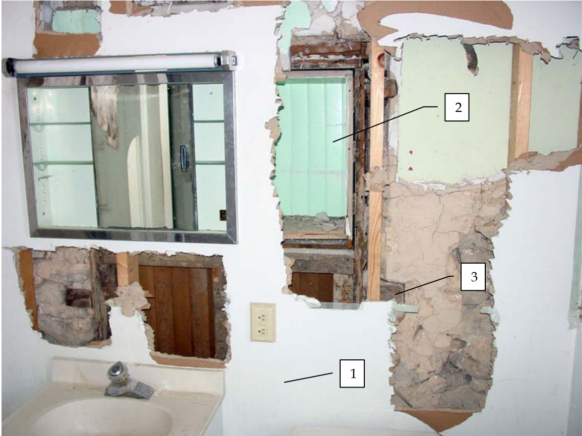
Photo 203a – View of west wall of Room 203, looking west. Former doorway between Rooms 203 & 207 located behind 20 th -century renovations.
