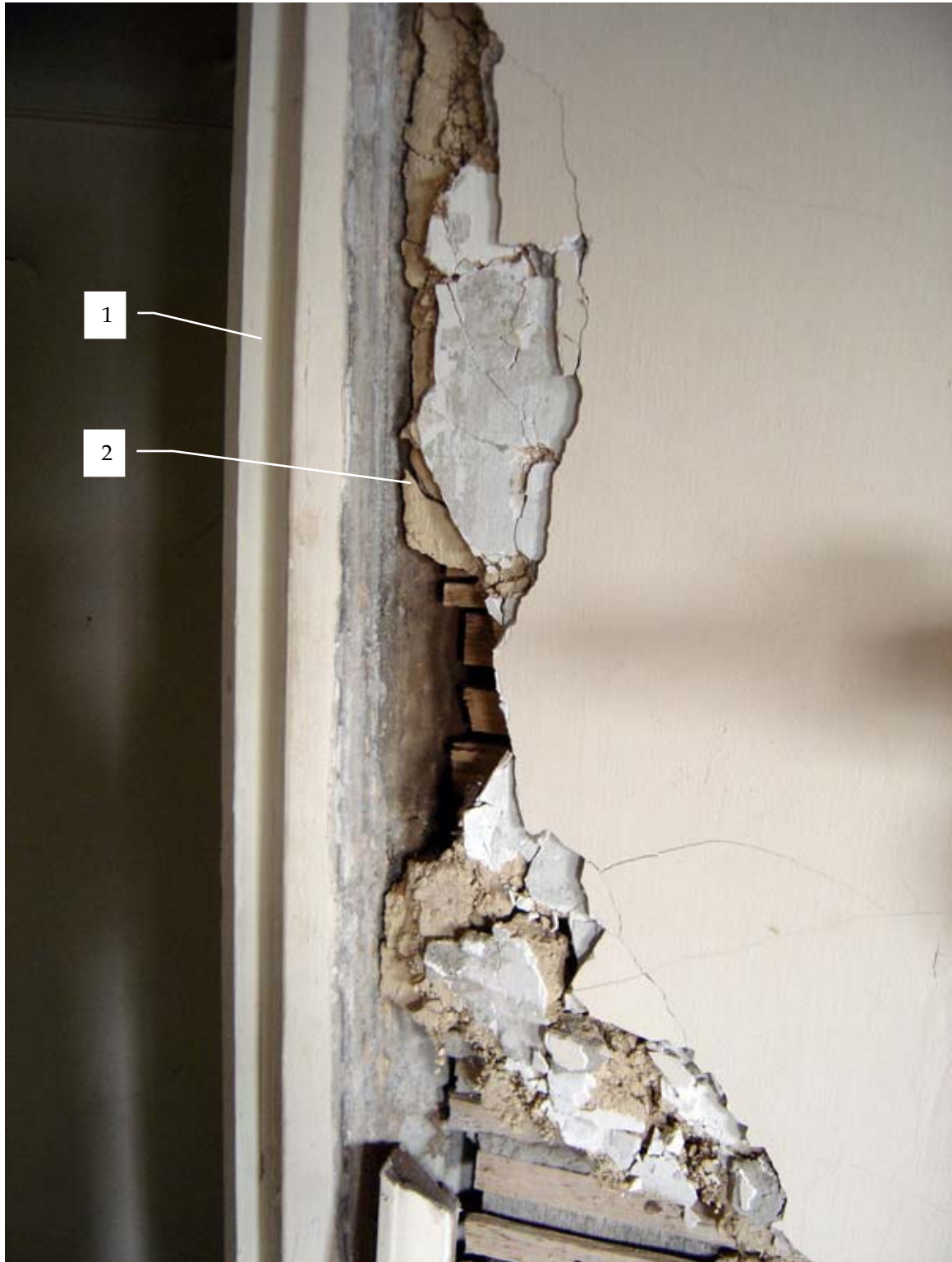
Photo 205b – Detail view of plaster at door jamb of closet, Room 205, looking northwest.
