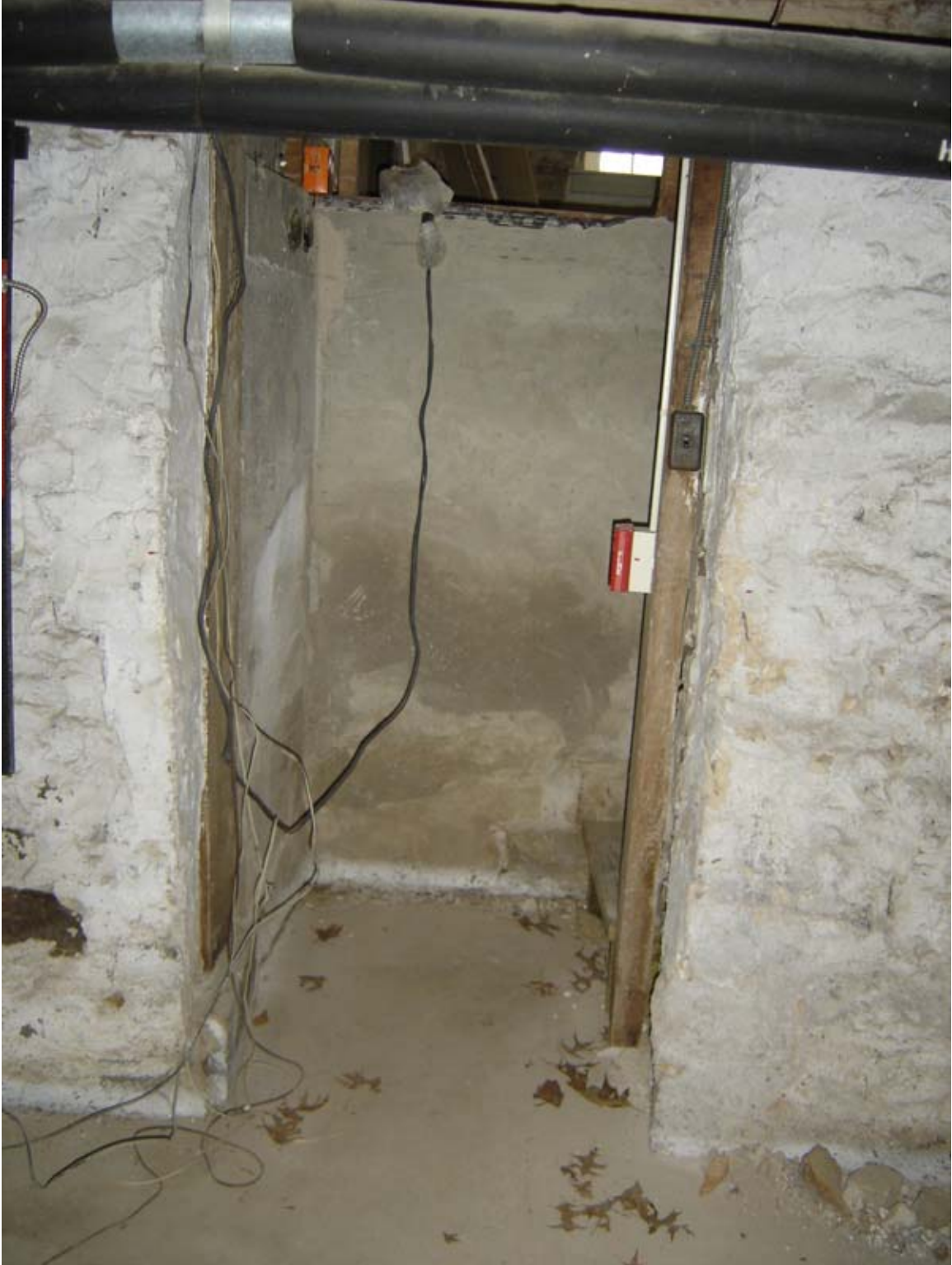
Photo 002d - Masonry opening at west wall, Room 002, looking west, into areaway for stair to Room 106. This opening was likely added as part of the c. 1926 alterations to the house to enable access to the basement from the first-floor kitchen.
