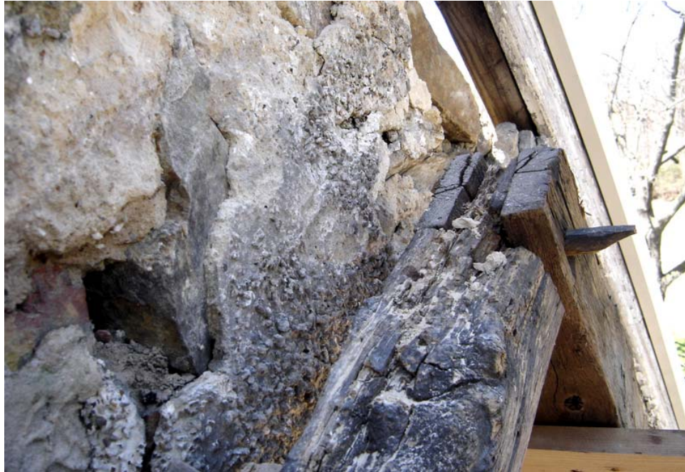
Photo EEb – Oblique view of east exterior wall of main block, looking northwest at location of east roof peak. Note that early lime-based stucco extends behind the east roof rafters. (East roof was removed at the time of this photo.) View represents the general location of Material Sample 14.
