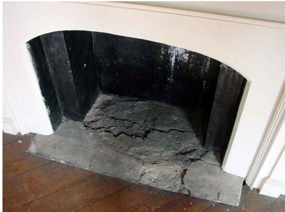
Photo 205d – Detail view of mortar hearth at corner fireplace, Room 205. Hearth is cracked and damaged.
