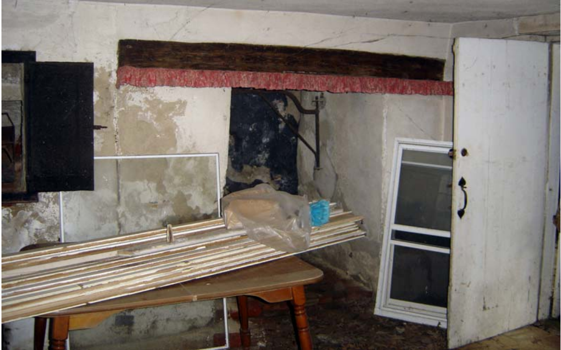
Photo 108a - Segment of east wall of bakehouse, Room 108, looking east. Fireplace has been modified substantially from its original configuration.
