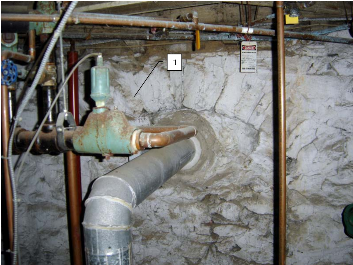
Photo 002a – Detail view of north fireplace foundation arch, Room 002, looking southeast. Alcove beneath arch has been infilled with stone and an exhaust flue from the current heating system has been introduced.
