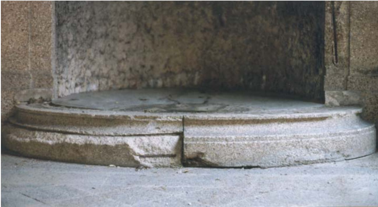
Fountain basin with missing lip and severe deterioration at main 16th Street entrance.
