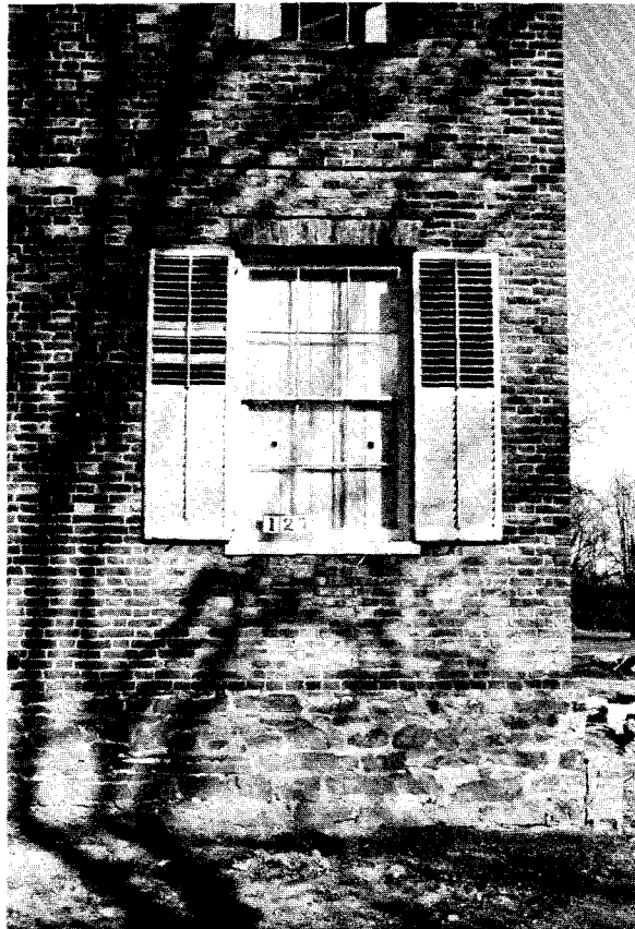
IP012, N012-08. Window 127, typical ca. 1797 window with ca. 1840 sash and shutter blinds.
