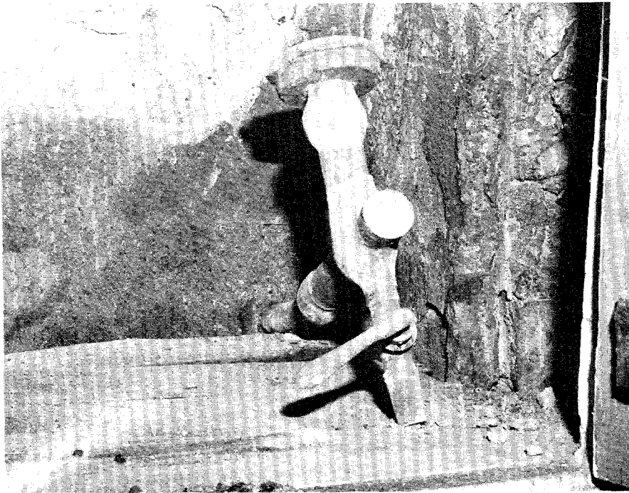
IP091, N038-01. Probable water supply to force pump, room 006, southwest corner at floor level.
