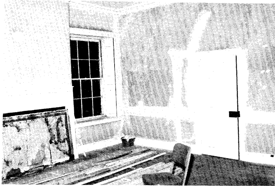
IP047, N030-15. Room 209, south and west walls. Note door 216 and its former location.
