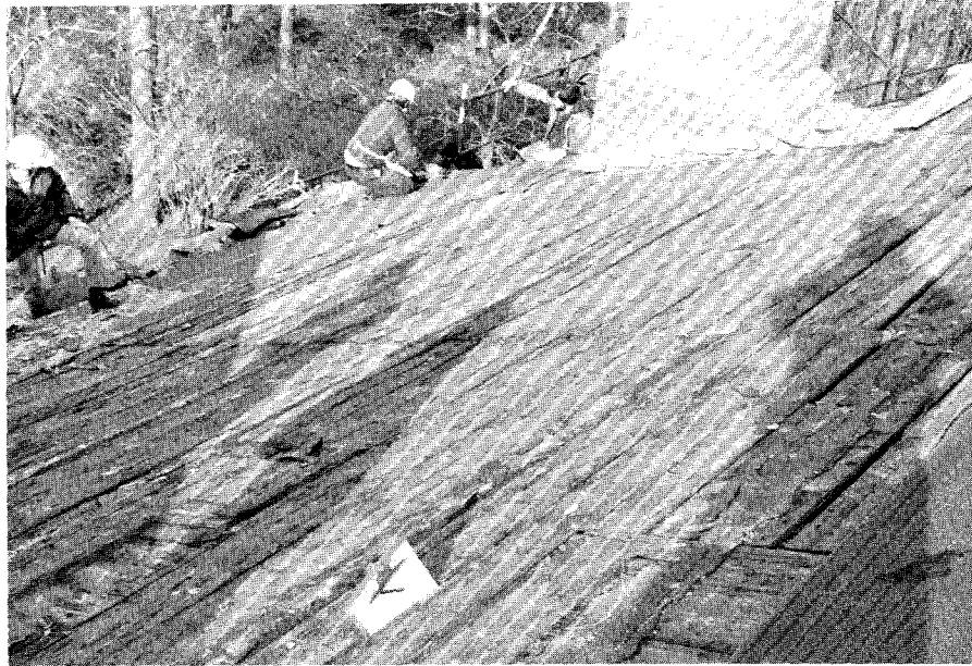
IP003, N039-01. Main roof, northwest corner looking northwest. Note hatch infill in foreground.
