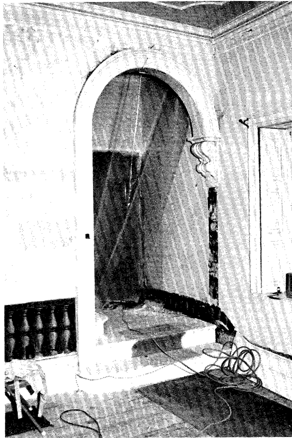
IP029, N022-12. Door 130 ca. 1849 alteration to room 105. Note patch in west wall about 8" above bracket.
