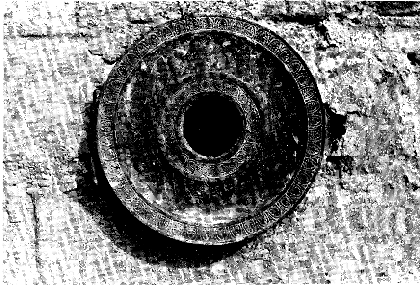
IP076, N015-16. Exterior cover for fresh-air intake duct.
