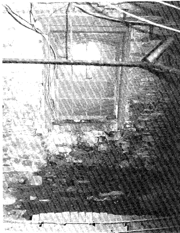
IP072, N028-35. Window 011. Note water penetration and dislodged masonry at lower left corner.
