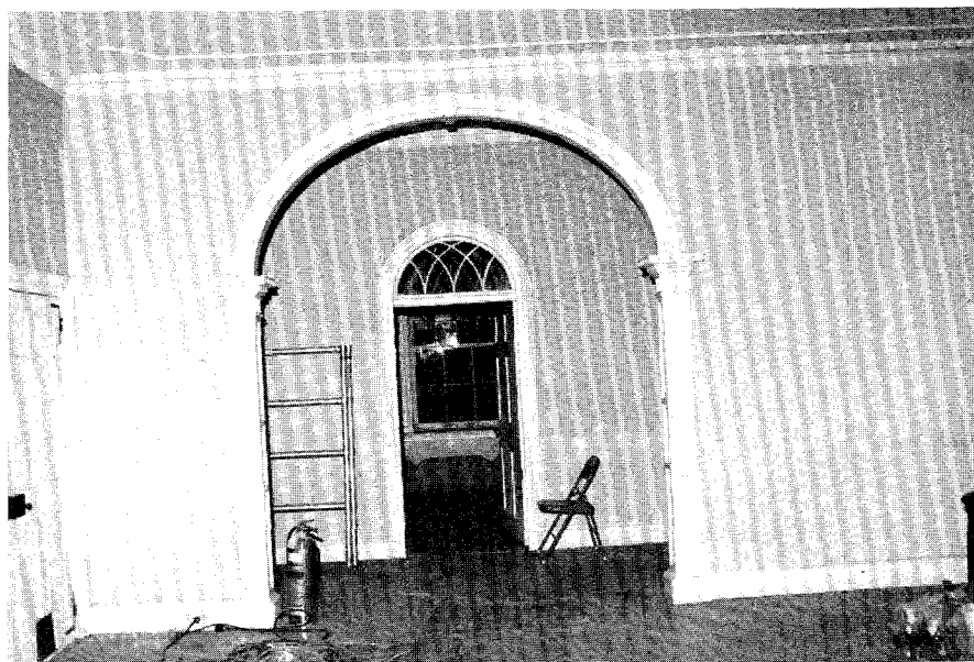
IP046, N030-03. Room 206, looking east into rooms 207 and 208 through doors 218 and 202. Note vertical line at former location of south wall near right edge.
