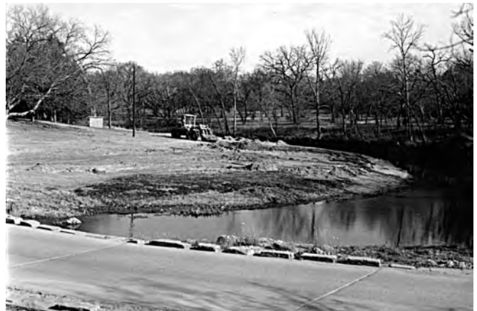
Figure 5-14. Regrading beach below Black Sulphur Springs after the flood of 1953.
