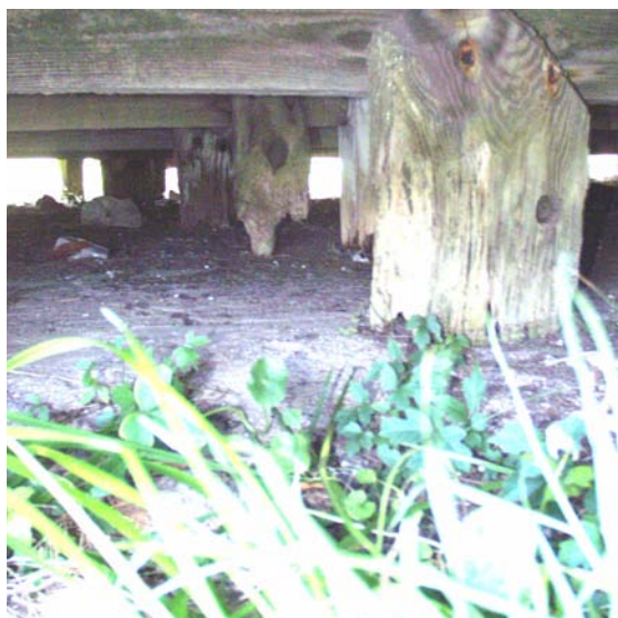
Figure 20 View of rotted wooden piers that formerly supported floor joists at mid-span. (NPS-SERO-CRS, 2002)
