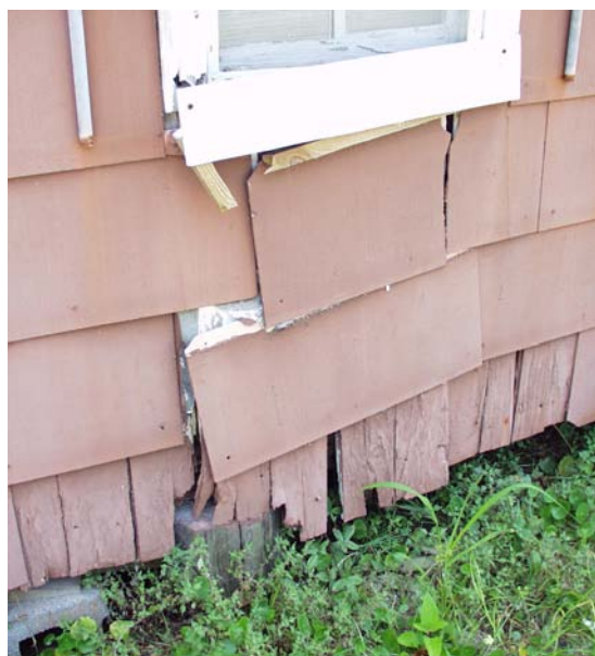
Figure 24 View of damaged siding on northeast side of house, the result of major sill damage in this location. Original board siding is exposed across bottom of wall. (NPS-SERO-CRS, 2002)
