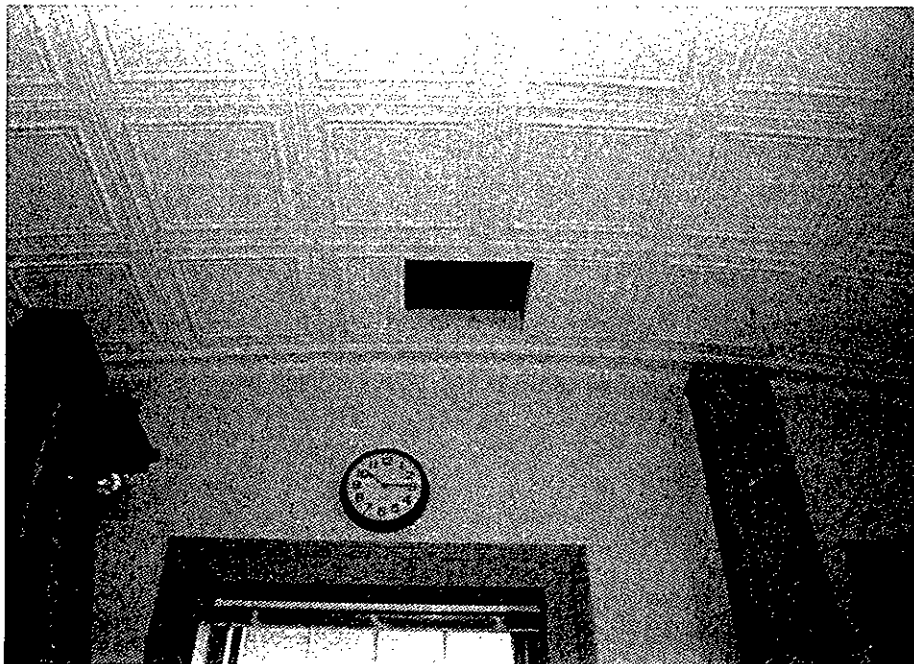
Figure 69. Smith School House: Second story, NPS office, ceiling and attic hatch at west wall (1990).
